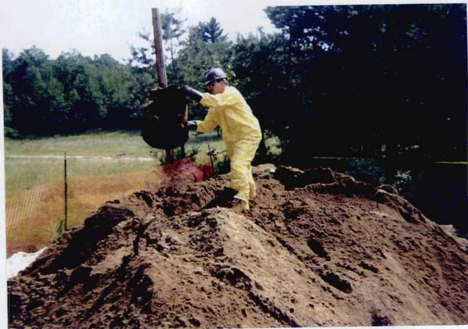
Photo 3 - MC Environmental Services worker removing drum from soil pile, Area D-1.
