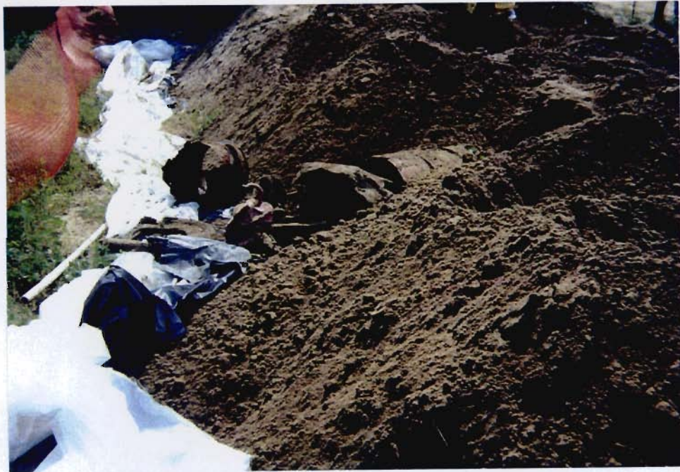
Photo 9 - Area D-1 soil pile and drum pile.
