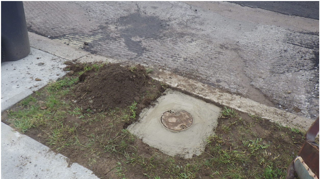
Picture 4: Raise Flushmount MW-05
