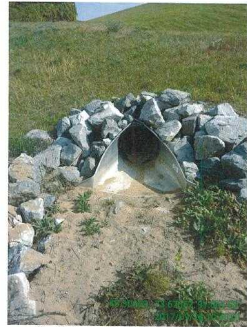
10 - Sediment Buildup at CB3 Outlet.jpg
