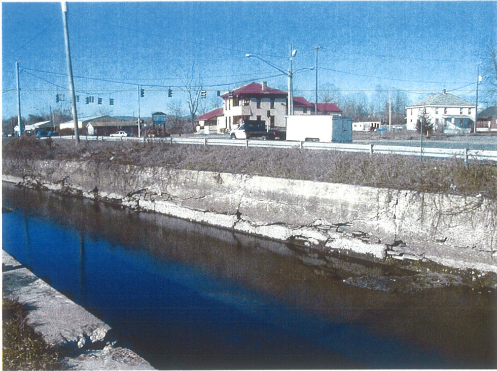
9. Deterioration in north wall of canal opposite intersection of Boulevard and Lower Warren St. (looking northwest).
