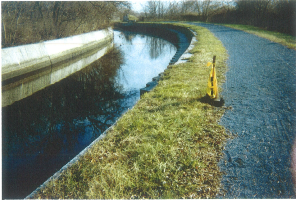
A3. Sinkhole between south wall of canal and towpath observed on 11/19/99 (looking east). Sinkhole is located on opposite side of the canal from the Sliver Quarry and a few feet west of the western end of the sheetpile repair work in the canal.
