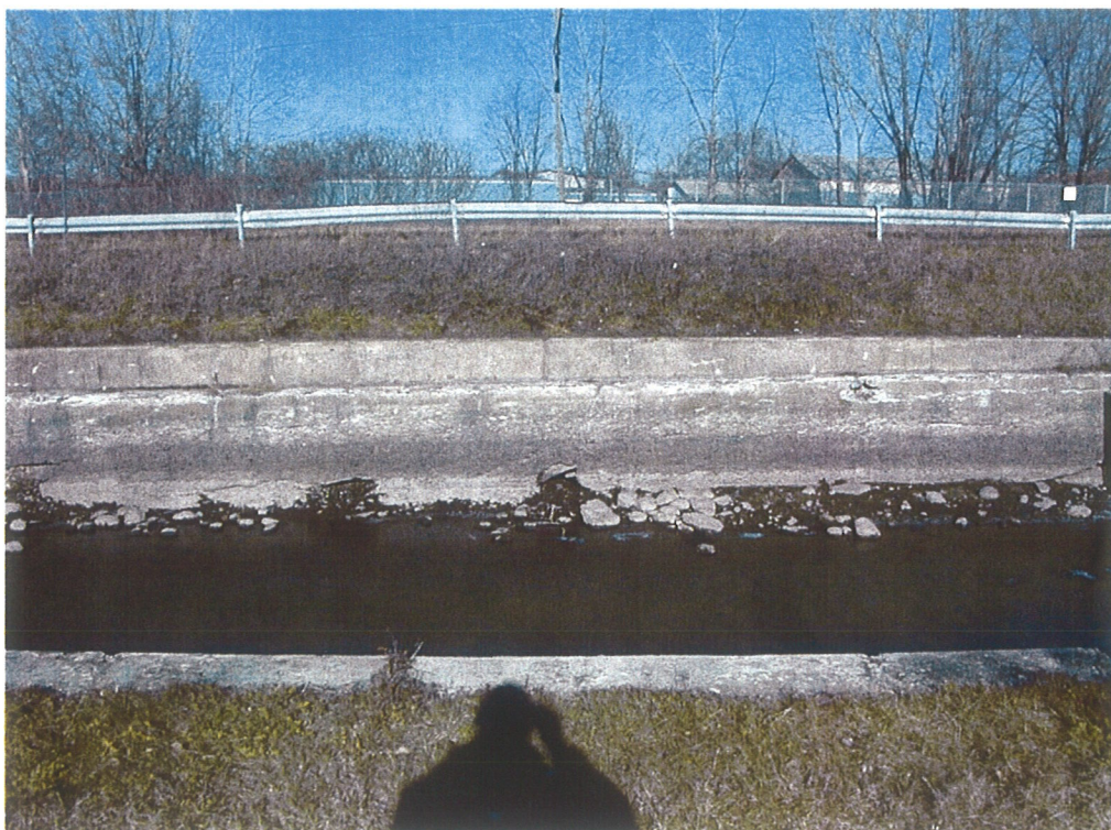
6. Deterioration in north wall of canal, opposite from middle of North Lot (looking north).
