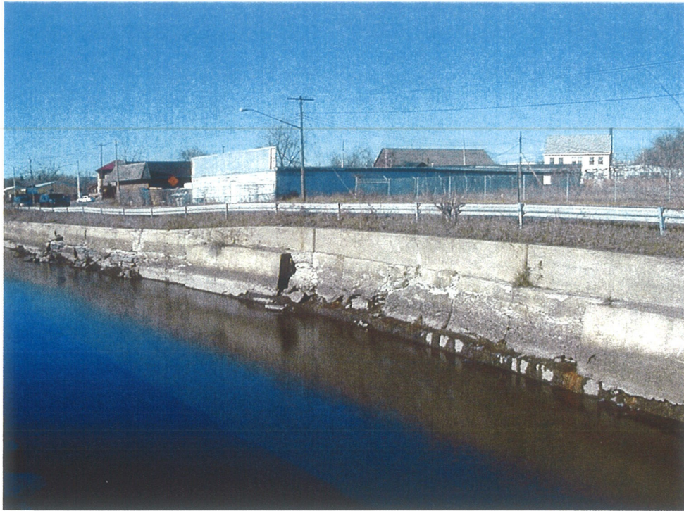
7. Deterioration in north wall of canal and local repair in wall, opposite west end of North Lot (looking northwest).
