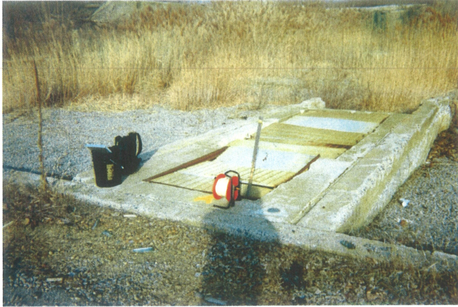
A5. Sump within foundation slab of former Building 5, designated as "Sump A".
