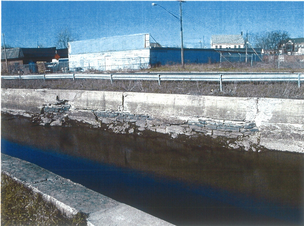
8. Deterioration in north wall of canal and local repair in wall, opposite west end of North Lot (looking northwest).
