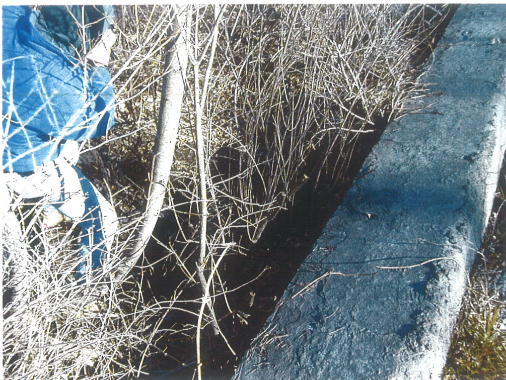
19. Sinkhole/washout in soil behind north wall of canal, approximately 15 feet east of sluice into canal (looking down to northeast).
