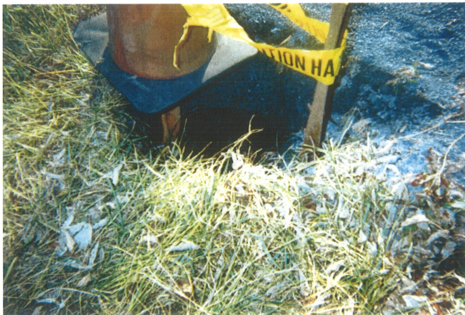
A4. Close-up of sinkhole in photograph A3.
