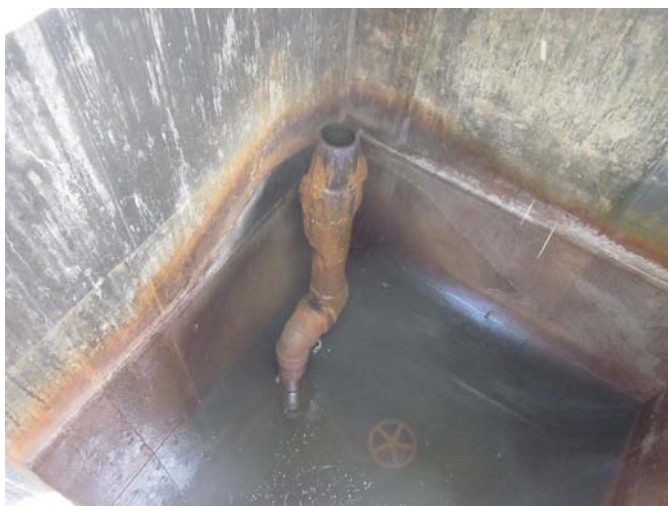
CWTS level control sump
