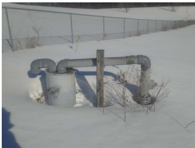
Typical CAP vent with bypassed carbon unit
