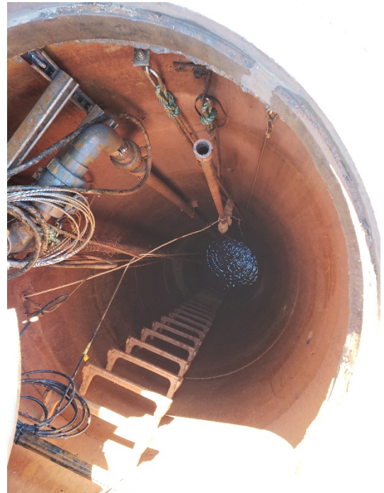
Figure 6 – Collection sump EW-4 - fall hazard and CSE
