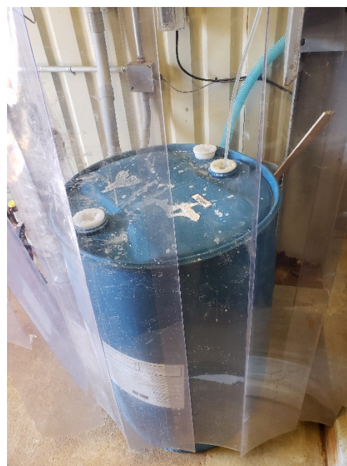
Figure 3 - Splash guard; some spillage noted.
