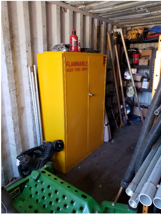
Figure 4 - Flammable storage cabinet.
