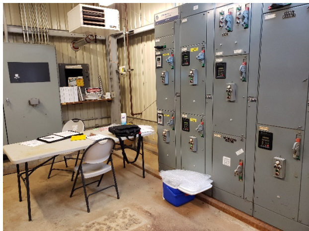
Figure 2 - Staging Area; electrical panels.
