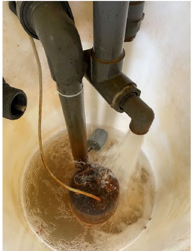
View of new decant tank float switch
