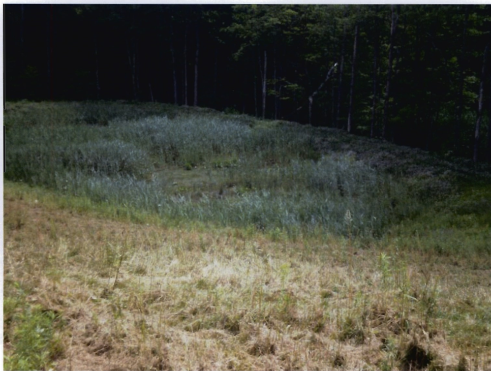
Photo 7: 7/12/2011-South Detention Pond with sediment accumulation.
