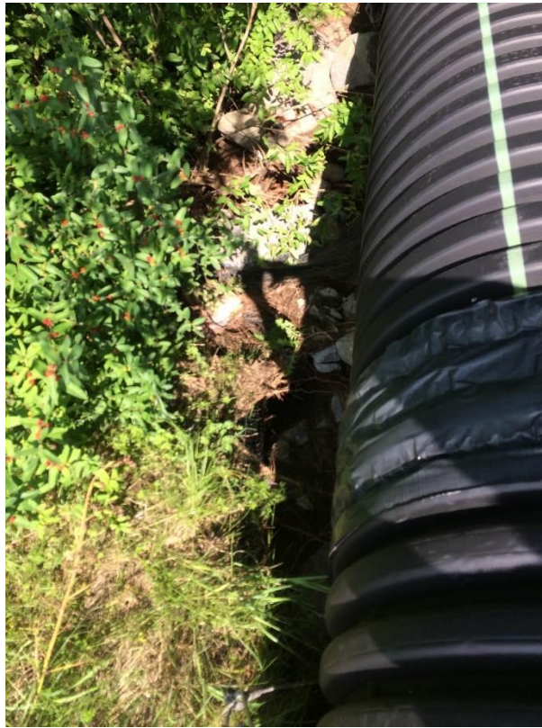
2015 Inspection – OSL Pipe Slope Drain #4 Failure 7/8/15 Erosion beneath Cell 2 pipe slope drain
