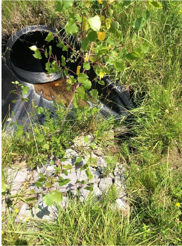
2015 Inspection – OSL Pipe Slope Drain #4 Failure 7/8/15 Inlet to Cell 2 pipe slope drain
