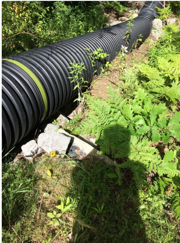
2015 Inspection – OSL Pipe Slope Drain #4 Failure 7/8/15 Cell 2 pipe slope drain
