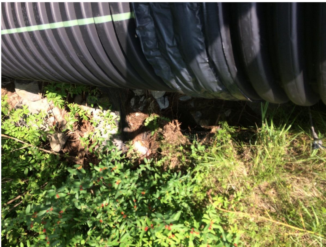
2015 Inspection – OSL Pipe Slope Drain #4 Failure 7/8/15 Erosion beneath Cell 2 pipe slope drain
