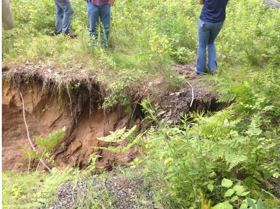
2015 Inspection – OSL Pipe Slope Drain #4 Failure 7/8/15 Slope damage at Cell 2
