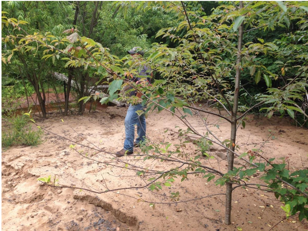
2015 Inspection – OSL Pipe Slope Drain #4 Failure 7/8/15 Deposition of slope sediments adjacent to OSL Creek
