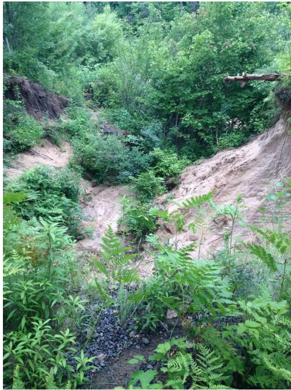
2015 Inspection – OSL Pipe Slope Drain #4 Failure 7/8/15 Slope damage at Cell 2
