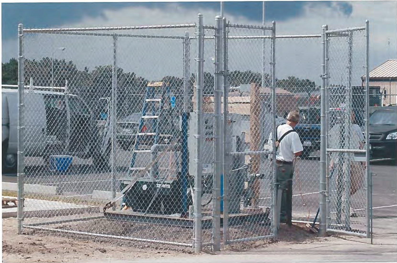
Photo 22. View of Completed Air Biosparging System Compound with 10-ft High Chain Link Fence
