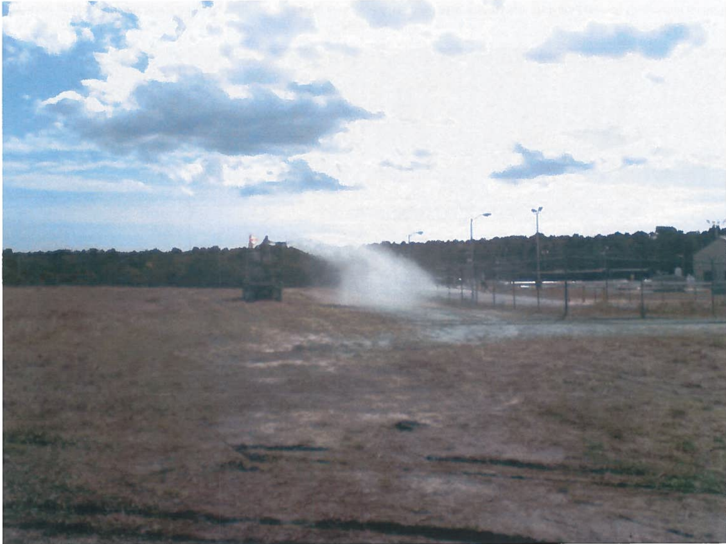
Photo 20. Active Hydro-Mulching of Main Air Supply Line Run with Water Cannon, Adjacent to POL Yard
