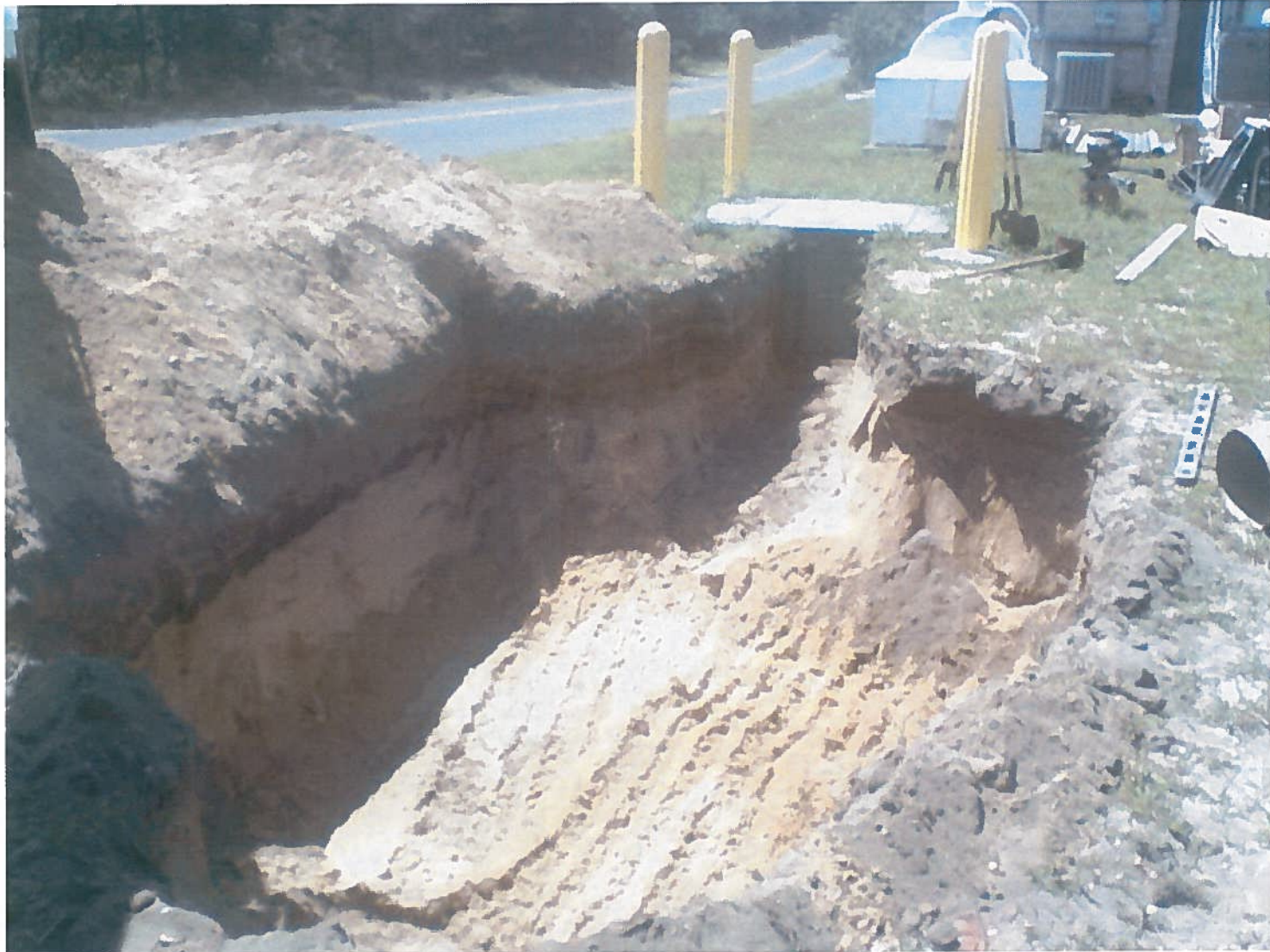
Photo 18. WRS Compass was Contracted by Electrician to Excavate Area for New Electrical Vault and Transformer
