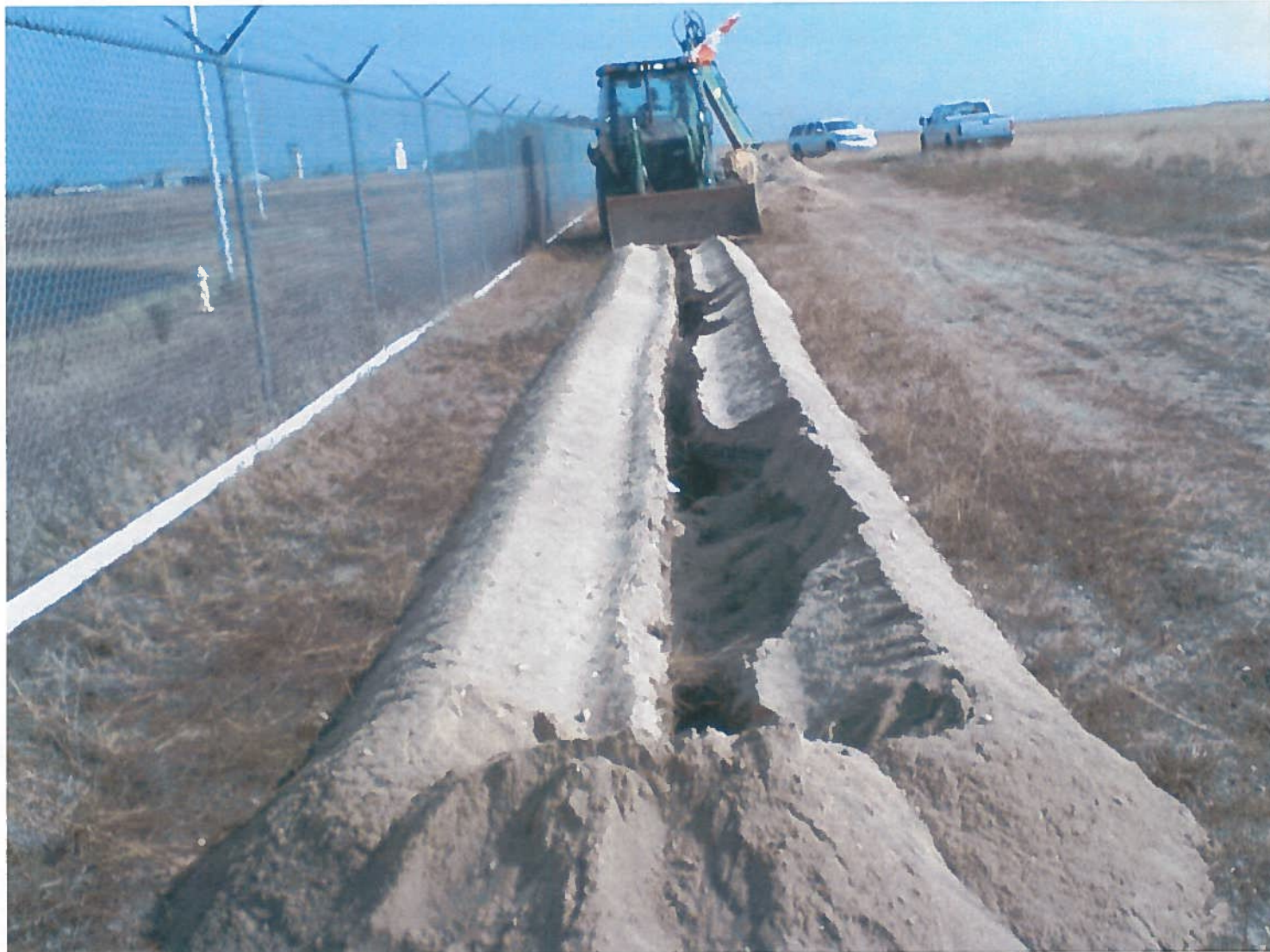
Photo 10. Sand Caved-In During Ditch-Witch Operation, Prompting Use of Backhoe to Install System Air Lines
