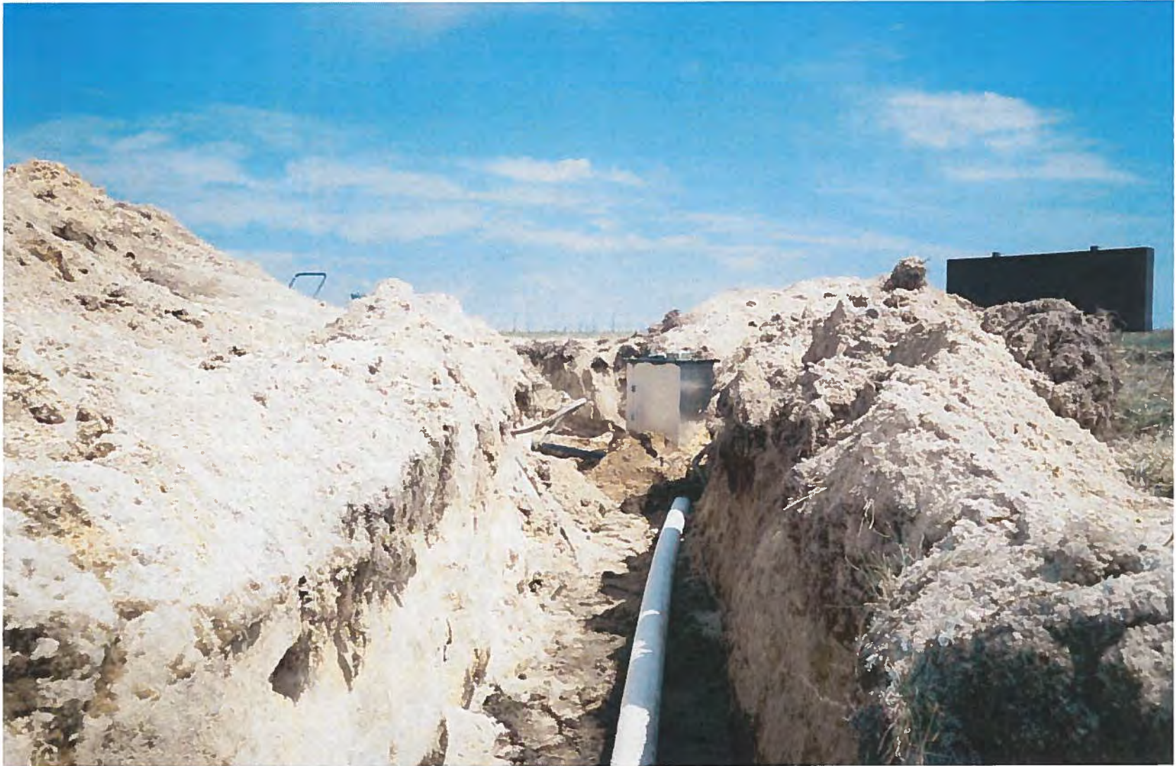
Photo 1. Installation of Main Air Supply Line and Main Vault Just Prior to Section Running Beneath High Speed Taxiway
