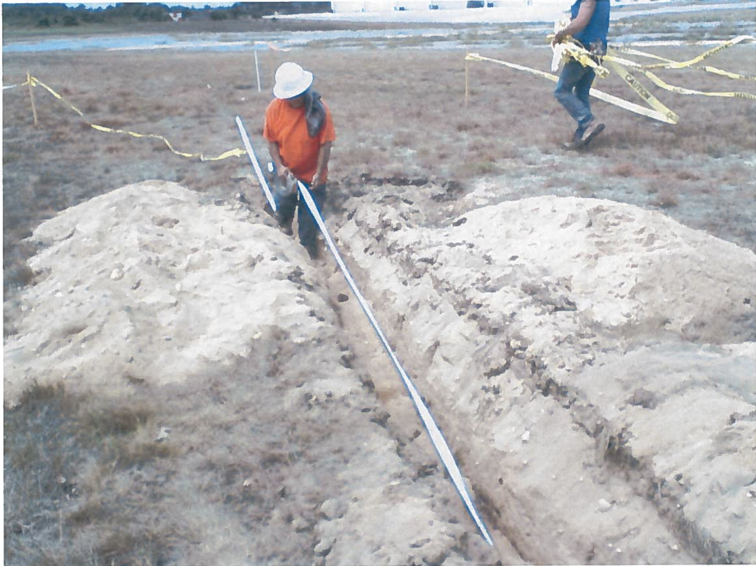
Photo 16. Installing Metal Utility Marking Tape to Facilitate Air Line Location with Metal Detectors
