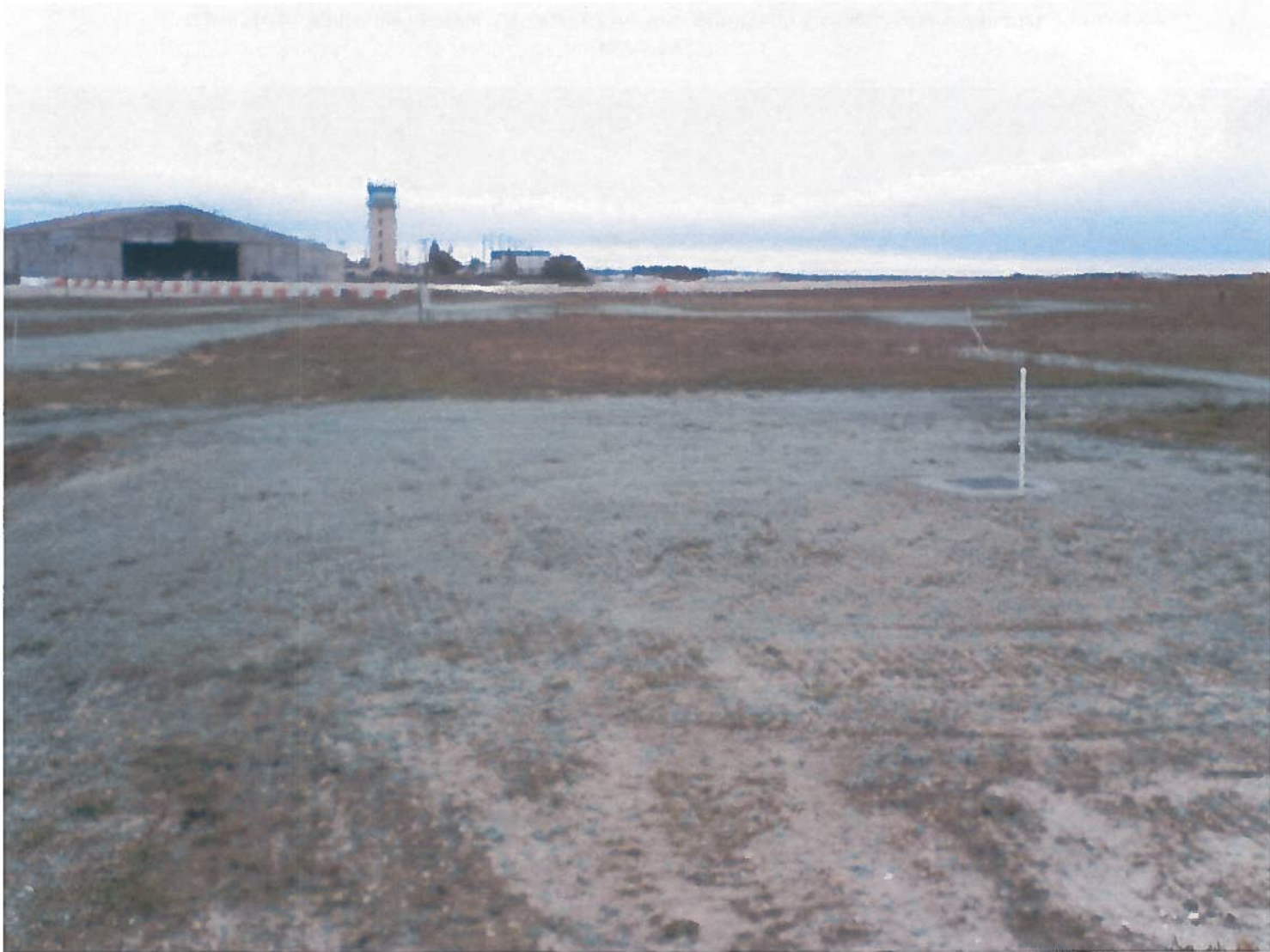
Photo 19. Site Restoration Included Mechanical Raking, Seeding with Gabreski ANG Seed Mix, and Hydro-Mulching (Green Coloration on Soil)
