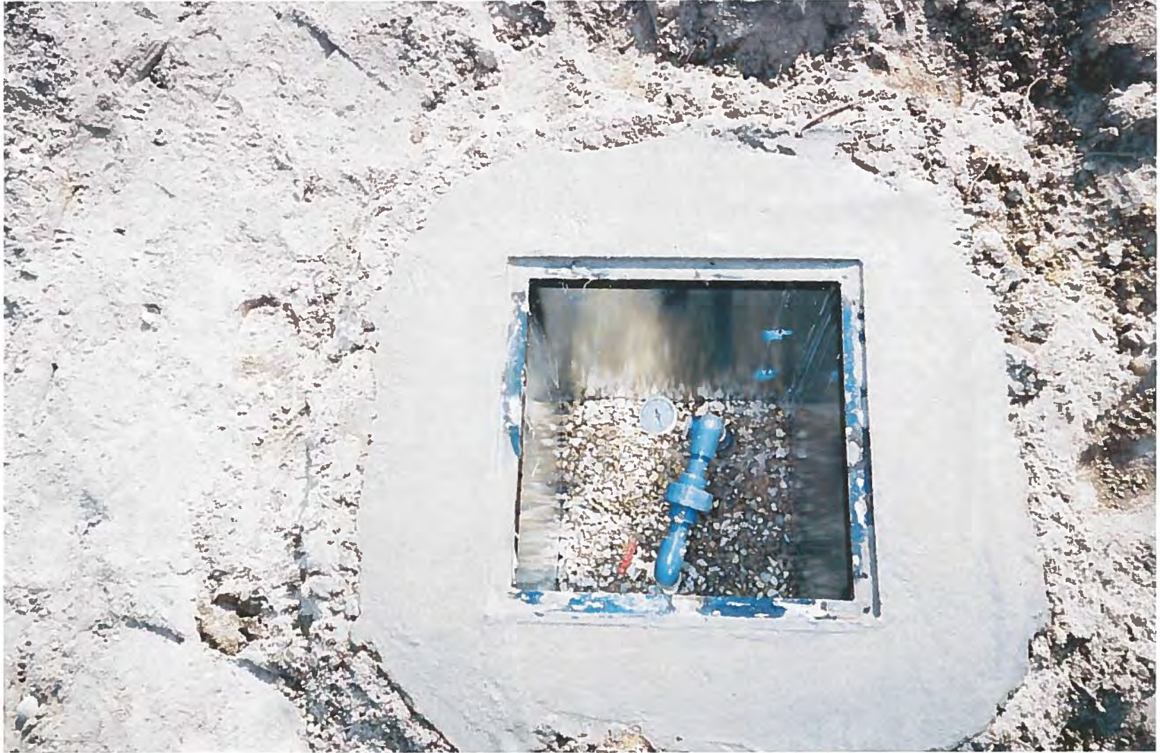
Photo 3. View of an Air Biosparging System Well Head With Pressure Gauge and Valve
