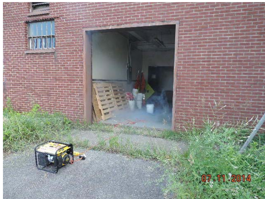
View of B817 smoke test smoke coming from floor drain to east of sump pit room.
