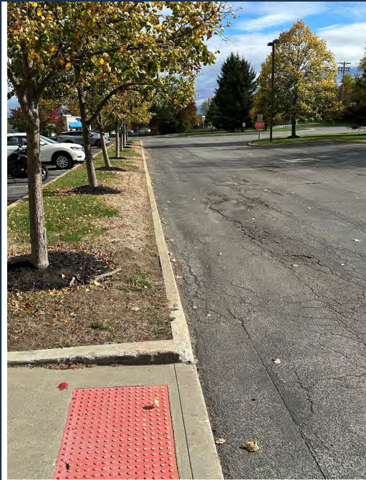
Photograph No.: 029 Comments: South side - East end showing typical pavement/landscaping - looking East.
