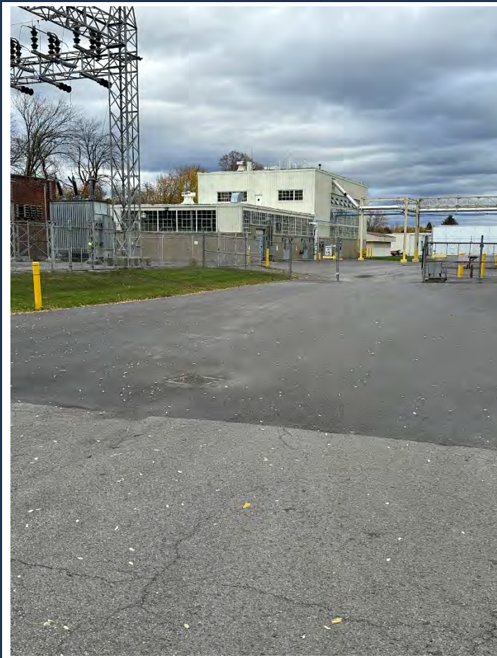
Photograph No.: 009 Comments: North side - West end showing electrical substation - looking Northeast.
