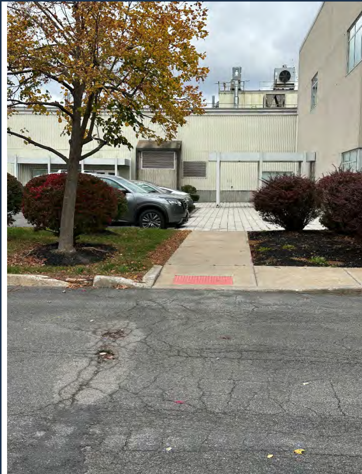
Photograph No.: 003 Comments: West side with sidewalk – looking North. Note minor pot holes.
