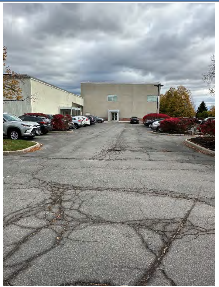
Photograph No.: 006 Comments: West side, typical parking area pavement – looking East. Note cracking of pavement.
