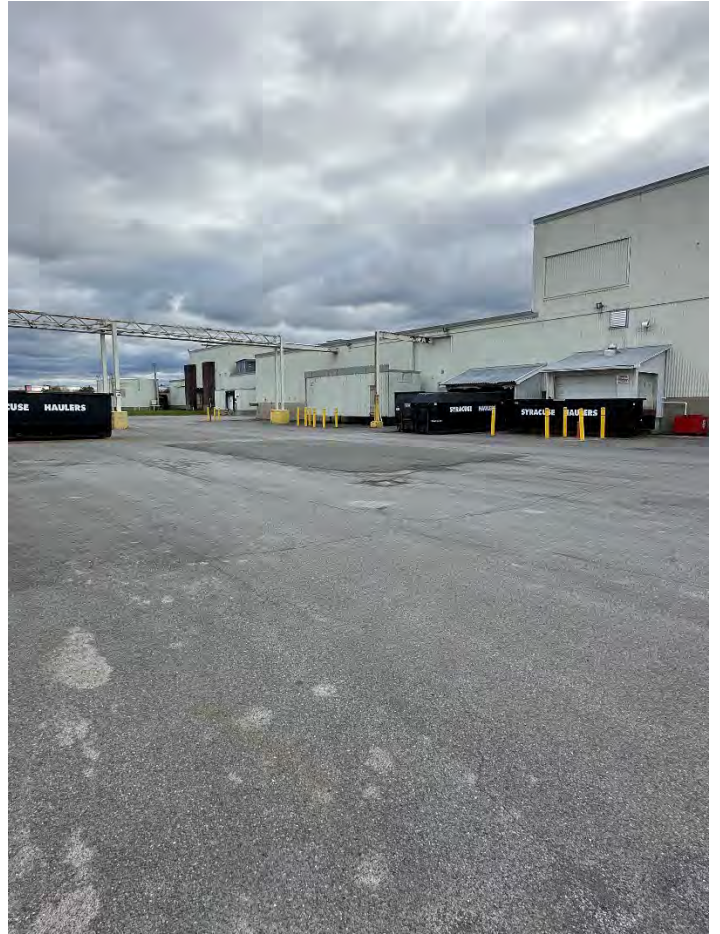
Photograph No.: 016 Comments: North side – Central area, looking Southeast. Note asphalt pavement repair.
