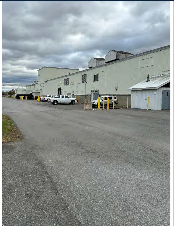
Photograph No.: 012 Comments: North side of West end of building showing March 2022 waterline repair area – looking West. Note asphalt pavement repair in area of water line repair.
