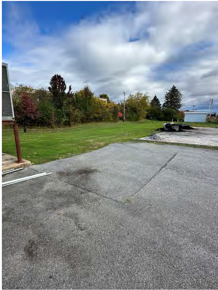
Photograph No.: 019 Comments: North side, showing East side of former pole barn concrete slab – looking Northeast.
