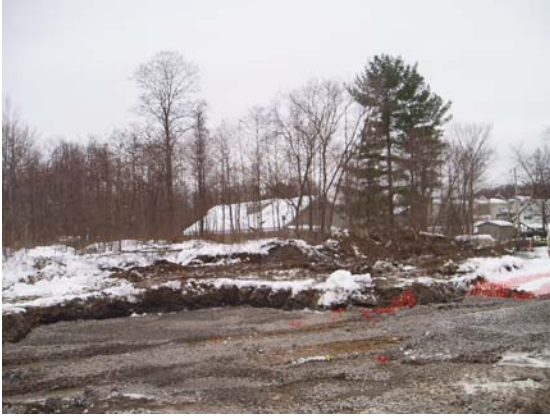
12/6/07 View of stone backfill in central portion of the three-foot IRM excavation area
