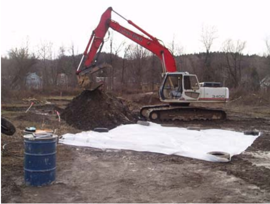
11/29/07 View of stockpiled PCB-impacted soil loading area looking southwest
