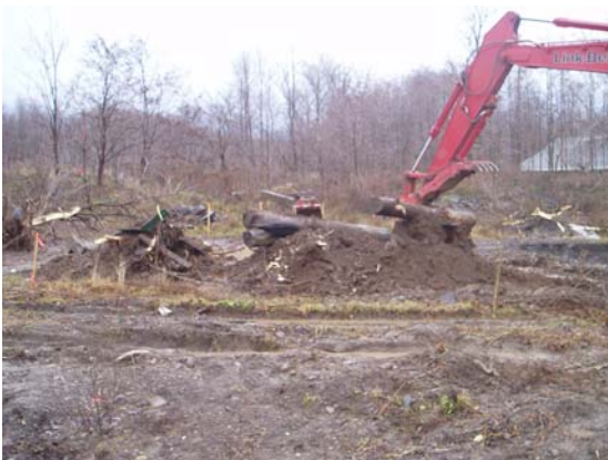
11/26/07 Logs and C&D debris excavated from the IRM excavation near the head of the Unnamed Ditch.
