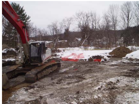
12/6/07 View of stone backfill in central portion of the three-foot IRM excavation area
