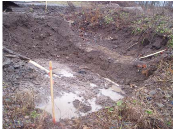
11/26/07 Water infiltration into the IRM excavation near the head of the Unnamed Ditch.
