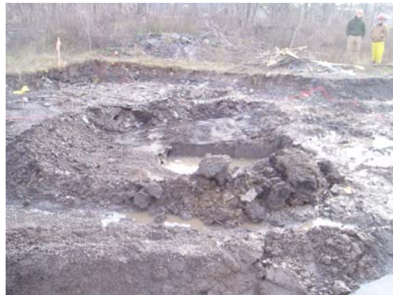
11/28/07 View of test pit at sample location SG-002 in the central portion of the IRM excavation
