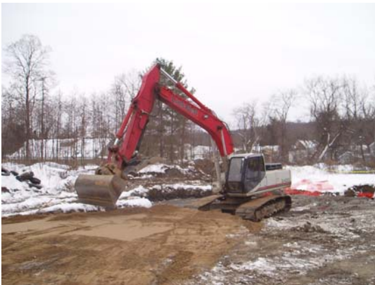
12/6/07 View of backfilling activities in the northeast portion of the IRM excavation
