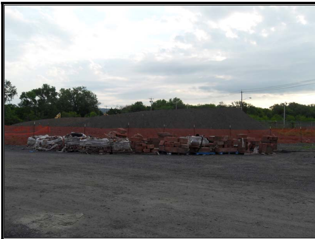
Photo #59: May 21, 2012 –Phase II: Excavation areas with water pools due to winter weather.
