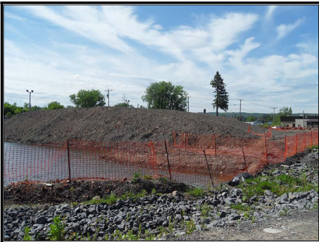
Photo #58: May 21, 2012 –Phase II: Excavation areas with water pools due to winter weather.
