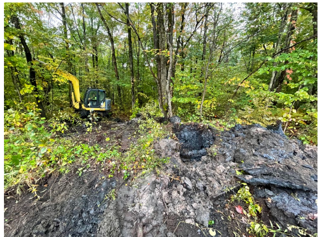
Photo 6: Surficial creosote in test pit E3.
