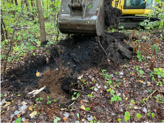
Photo 7: Surficial creosote in test pit E10, observed approximately 1 to 2 ft bgs.
