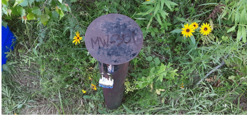
MW-301 Protective Casing
