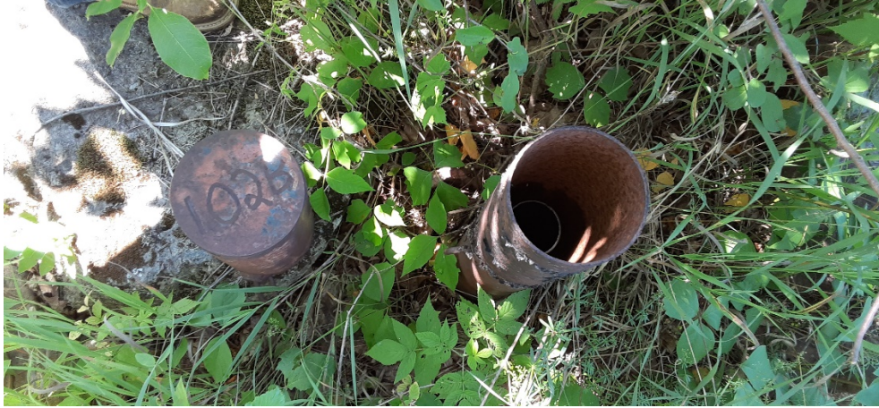
MW-102B Protective Casing and Monitoring Well
