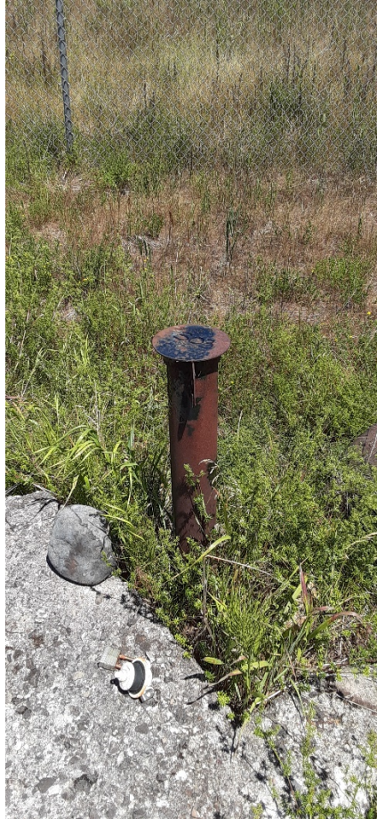
MW-303 Protective Casing
