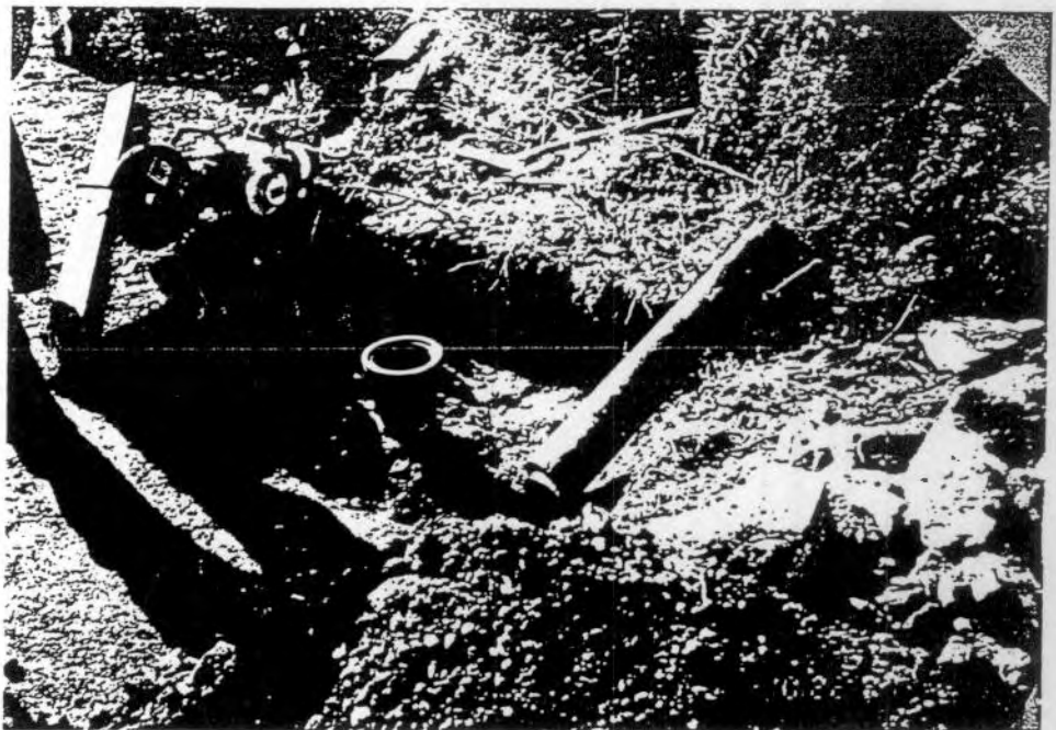
MW-1 cut down to grade prior to new apron and manhole cover installation.
