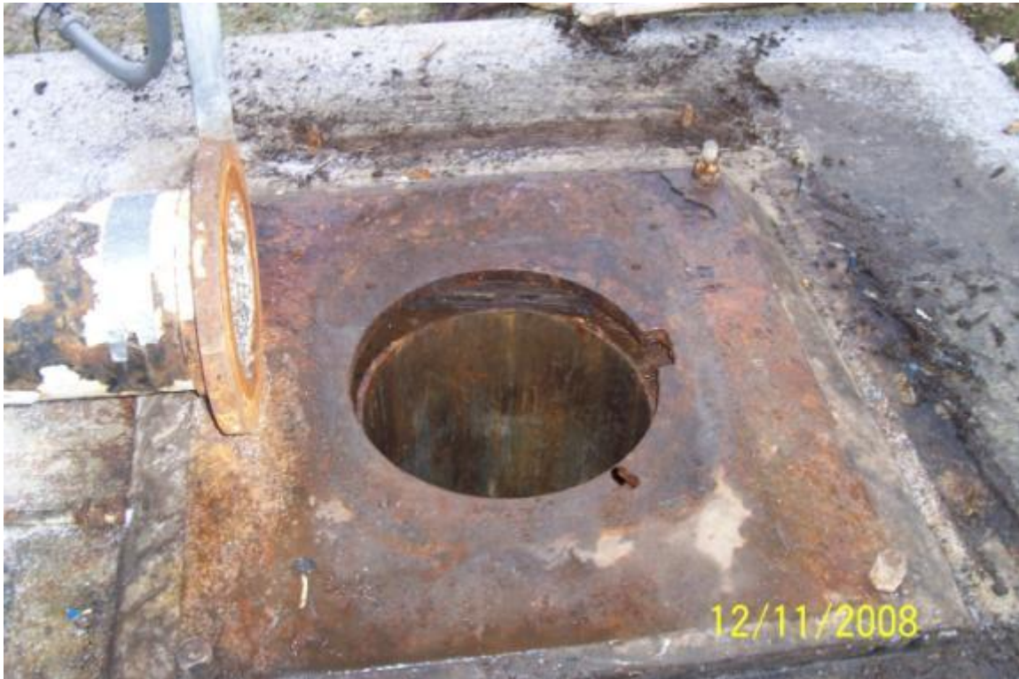
Photo 13: Line-shaft pump motor support pad
