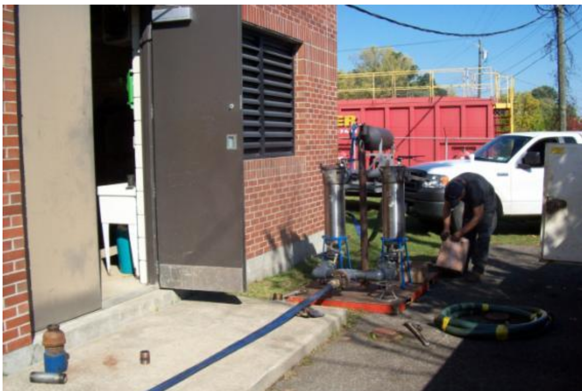
Photo 10: Bag filtration system
