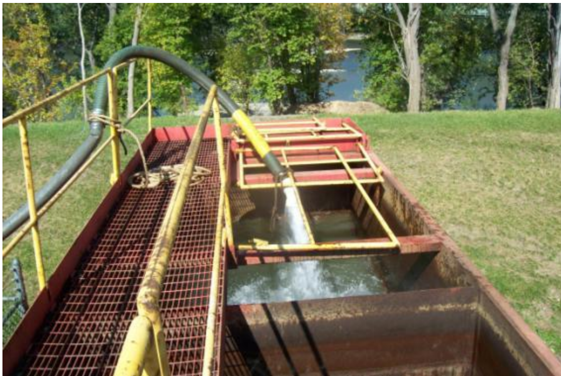
Photo 9: 12,000 gallon temporary storage container for well development water
