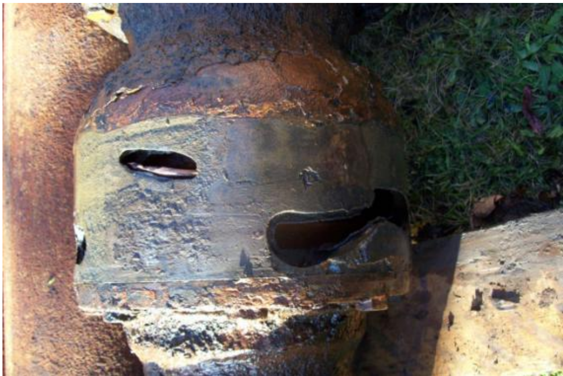
Photo 2: Severe corrosion on pump bowl assembly
