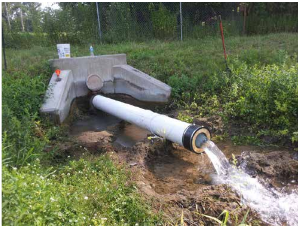
Discharge Orifice Installed at Well 1-1A Treatment Plant Outfall
