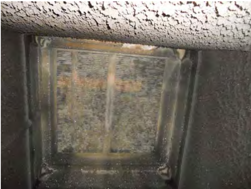
Media support screen at base of air stripper tower.
