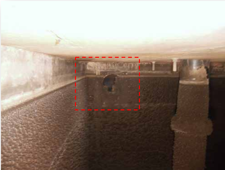
Obstruction in 12" clear well outlet pipe.
