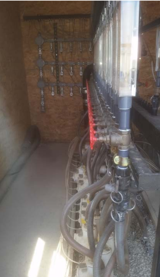
Picture 8 - Distribution Cell 2 Interior
