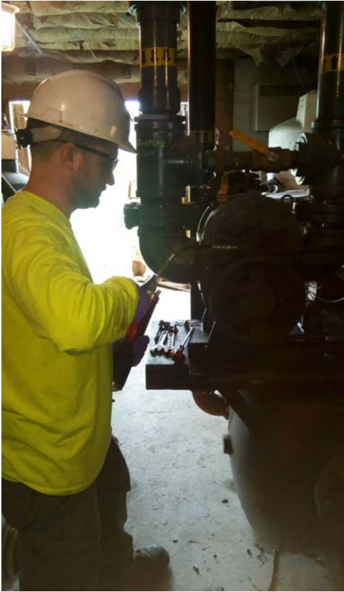
Picture 3 - Greasing the Injection and Vacuum Blowers
