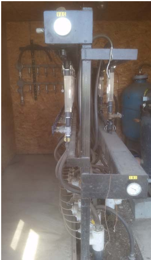
Picture 6 - Distribution Cell 1 Interior
