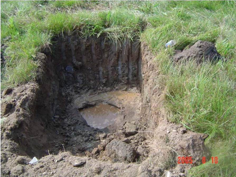
COLE-2 Investigation Location Standing Water in Drainage Layer Above Liner
