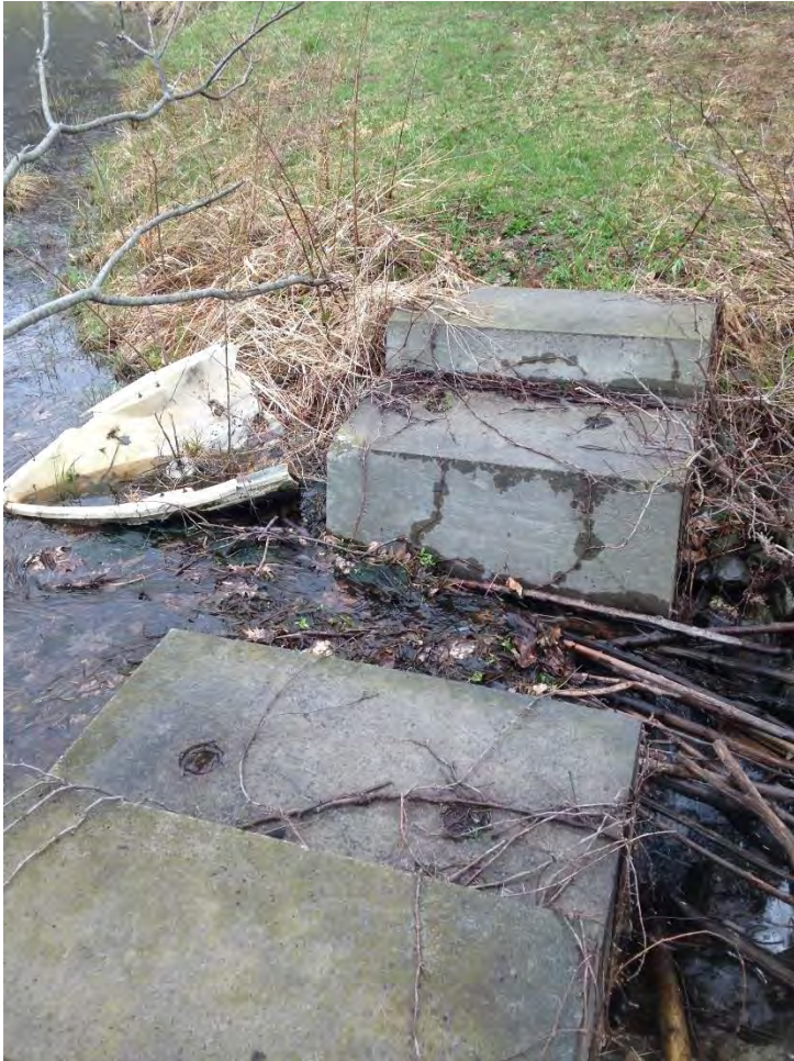
ABP Discharge Structure (blocked) 4/23/15
