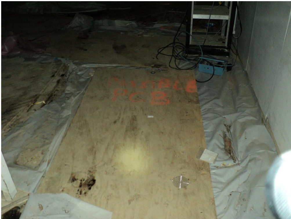
PCB Contamination in Production Building
