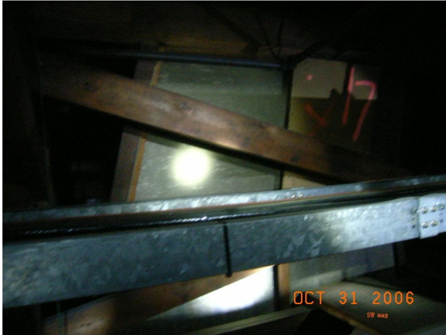
Transite Duct above Catwalk
