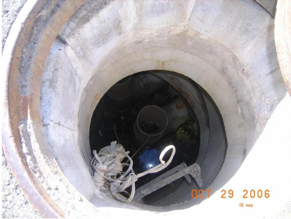
Oil Water Separator near Exit 10
