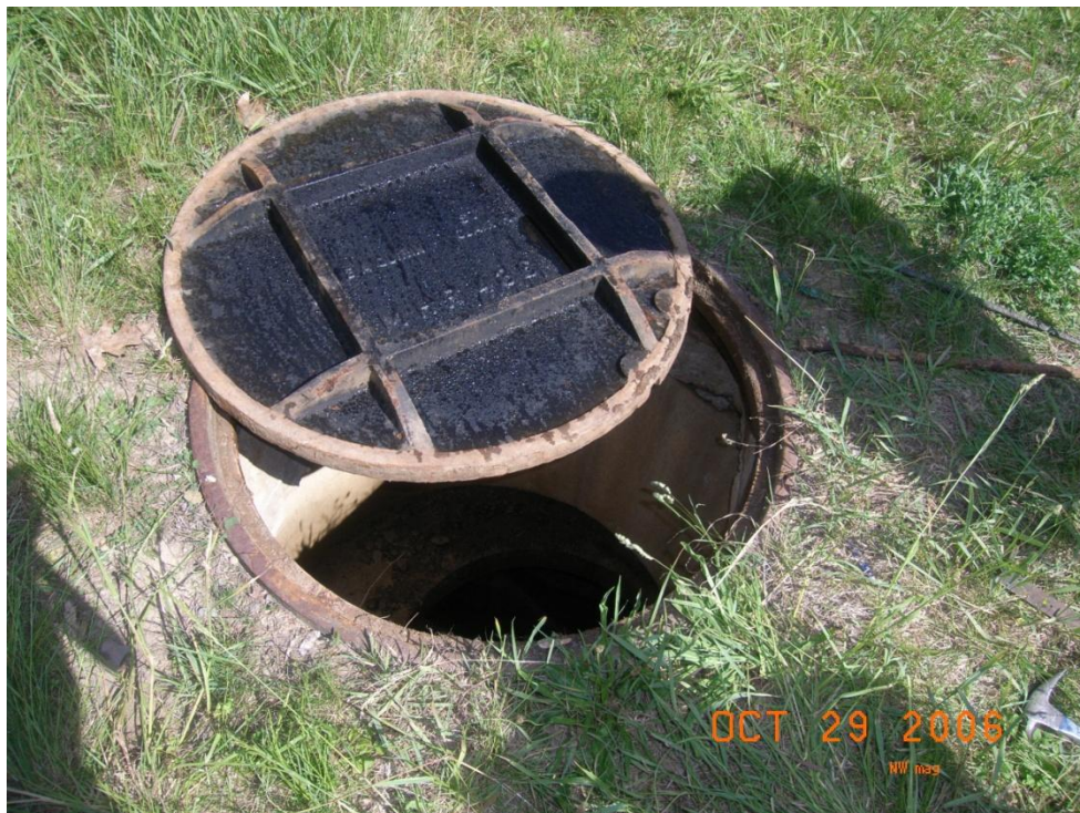
Oil Water Separator near Pump House
