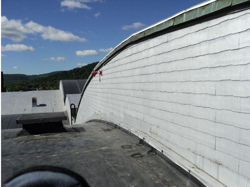
Asbestos Shingles on Roof
