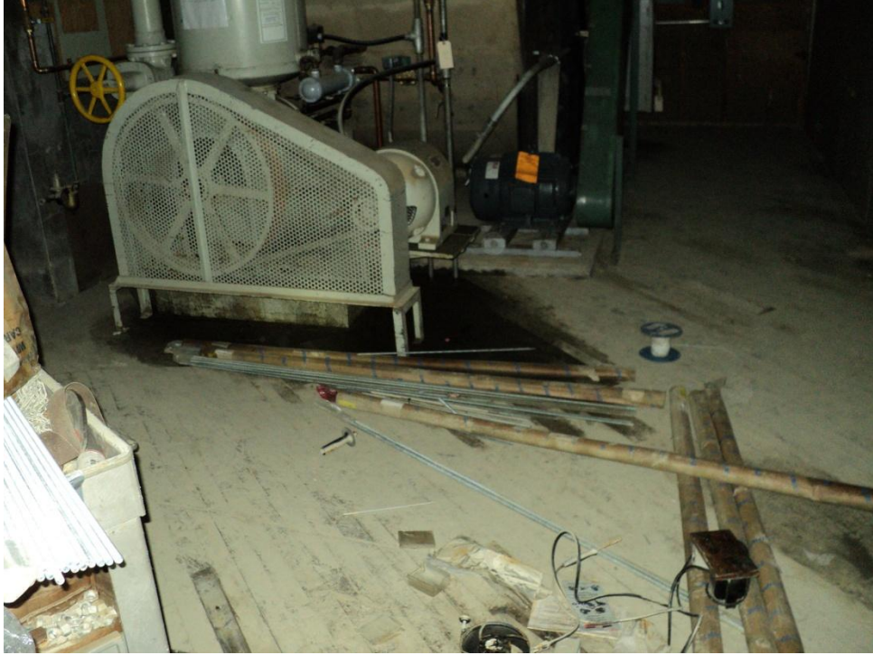
Oil Contamination on Floor of Production Building
