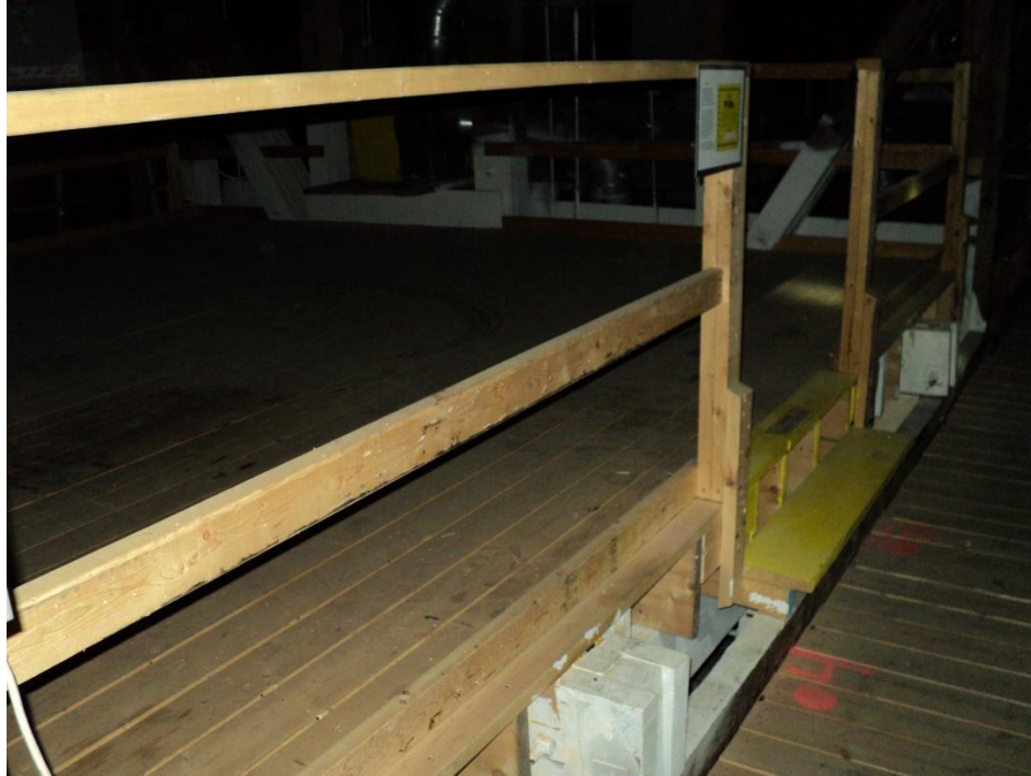
PCB Contaminated area in Catwalk (Posted)
