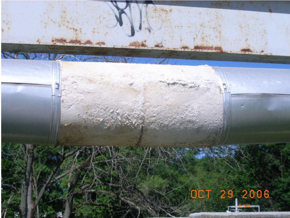
Steam Pipe (Metal Jacket Fallen Off)
