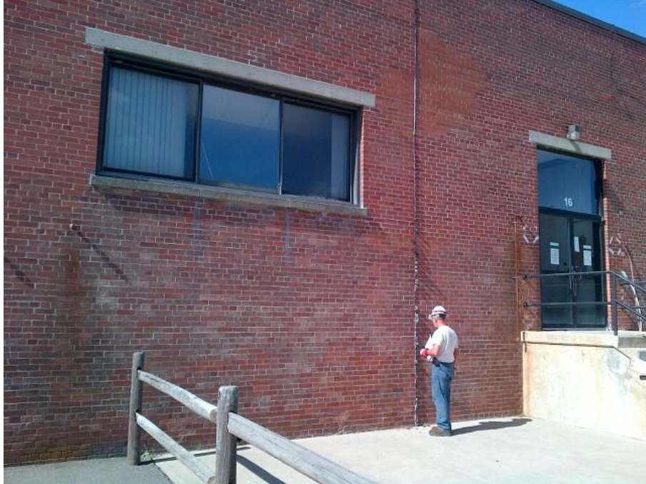
Wall Sealant (Suspect ACM) near Exit 16
