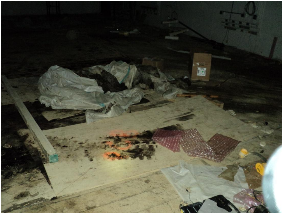
Oil Contamination on Floor of Production Building
