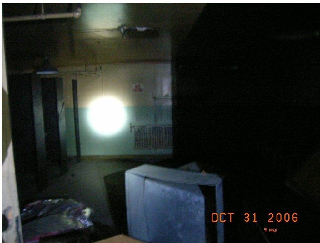
Very Large AHU, North Catwalk (Posted PCB Contaminated)
