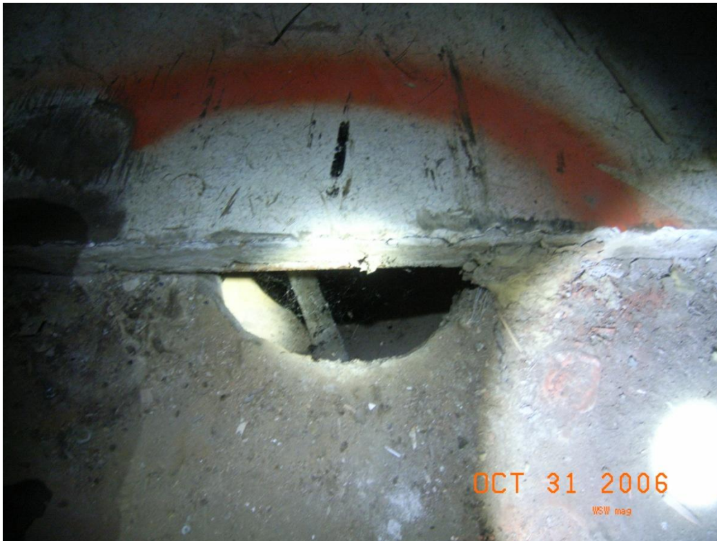
Hole in Floor (Part of Metal Reclamation Unit) Production Building
