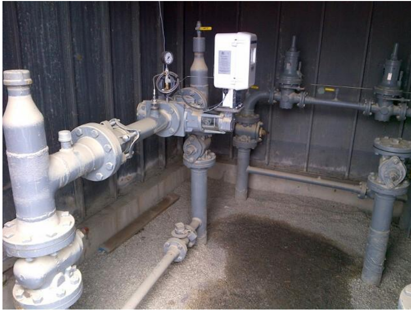
Oil Staining in Natural Gas Pipeline Shed, East Parking Lot
