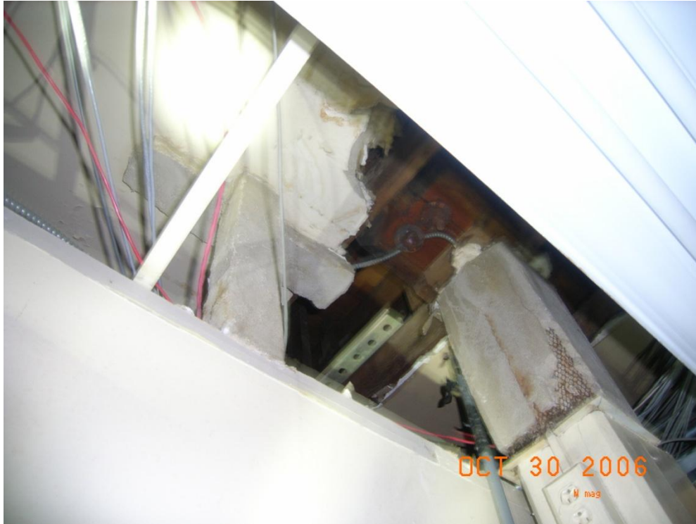
Suspect ACM on Beams & Some Columns Office Bldg & Production Bldg
