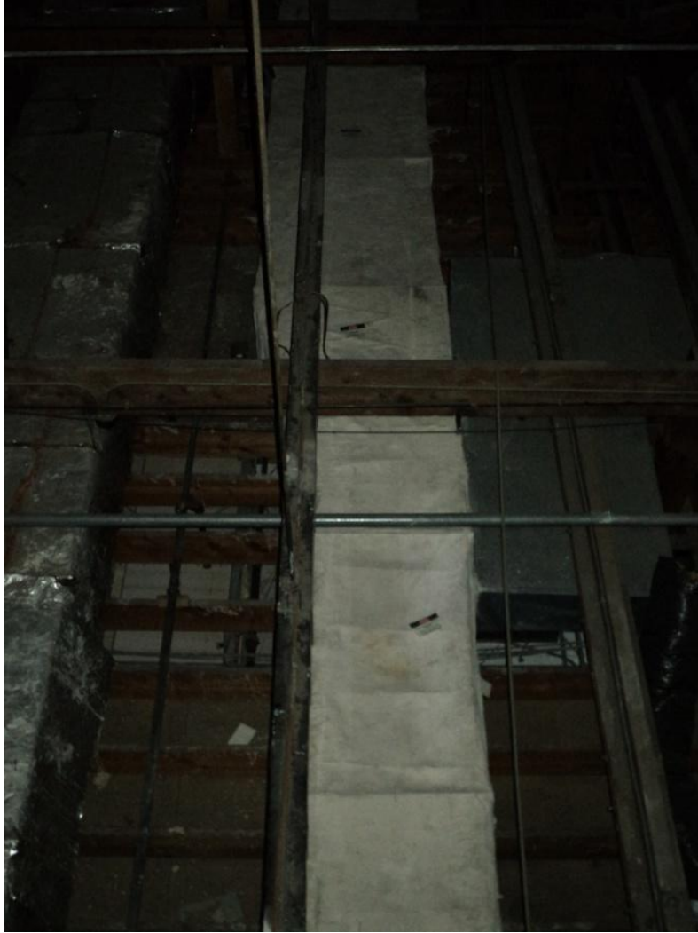
Duct Insulation – Catwalk (Labeled ACM-containing)
