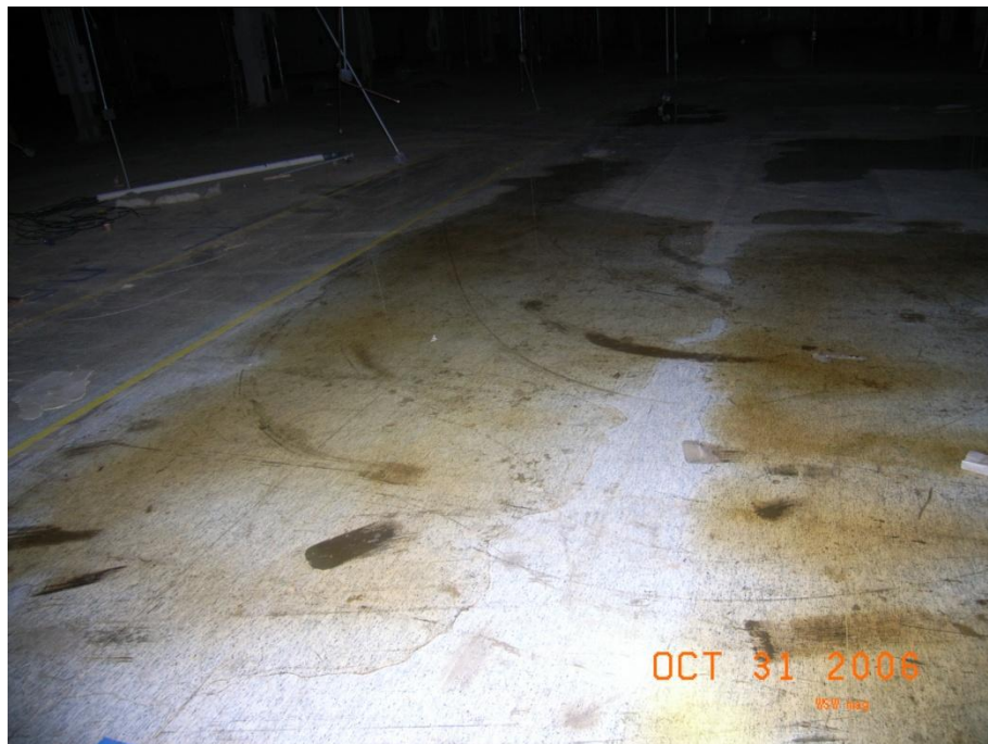
Staining of Floors in the Production Building
