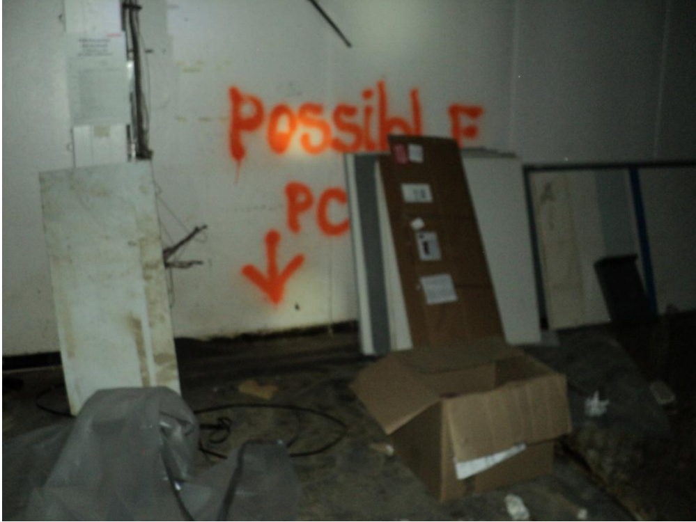
PCB Contamination in Production Building
