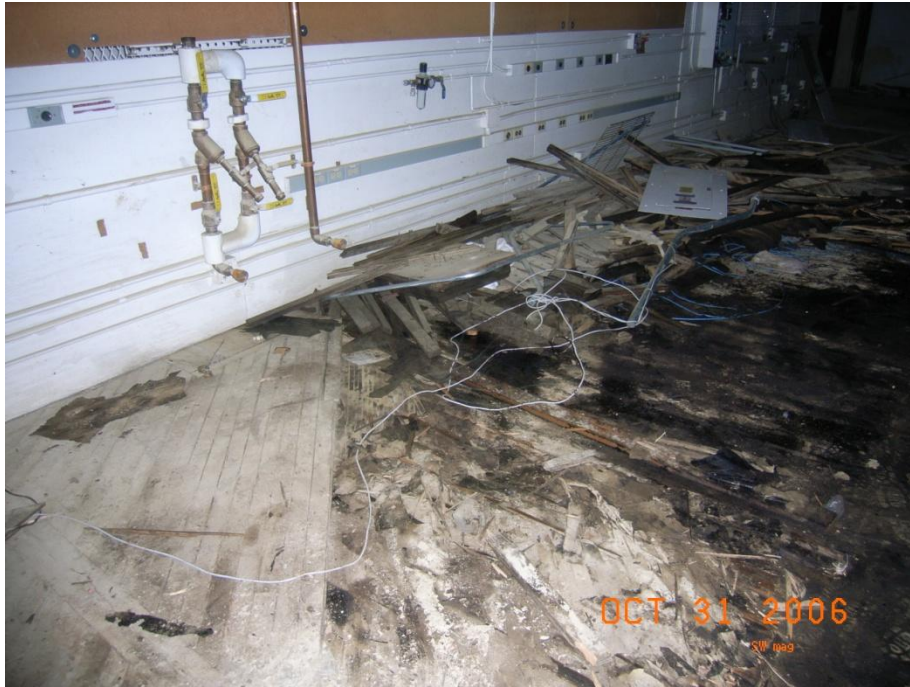
Oily Substance on Floor (Wood Planks removed) Room 703
