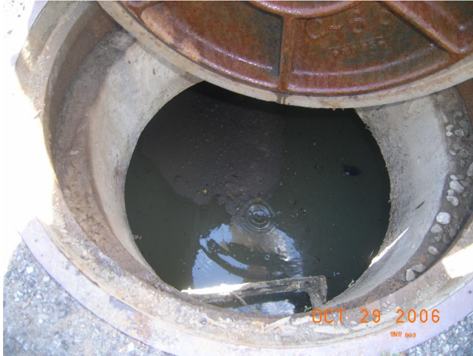
Oil Water Separator North Parking Lot
