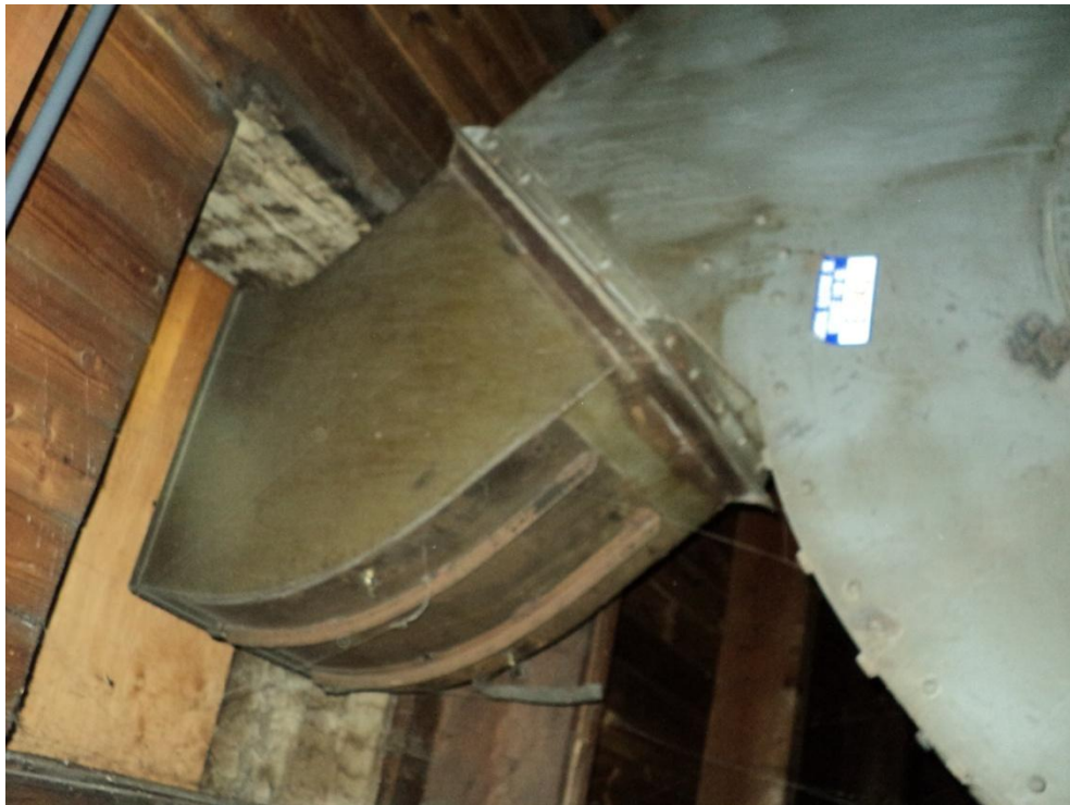
Metal Reclamation Unit in Catwalk
