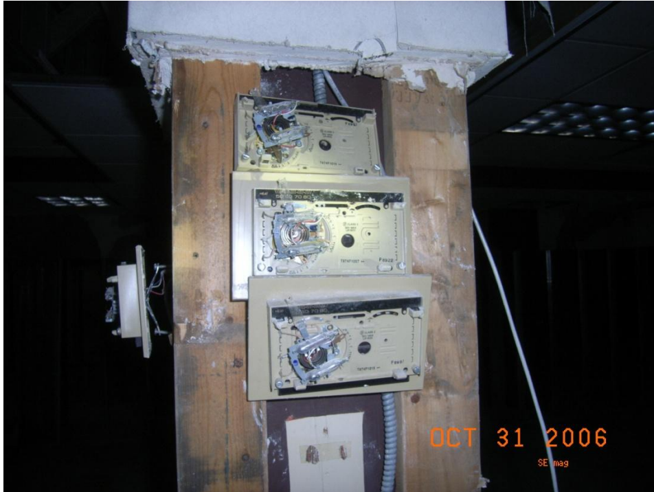
Mercury Thermostats in Office Building
