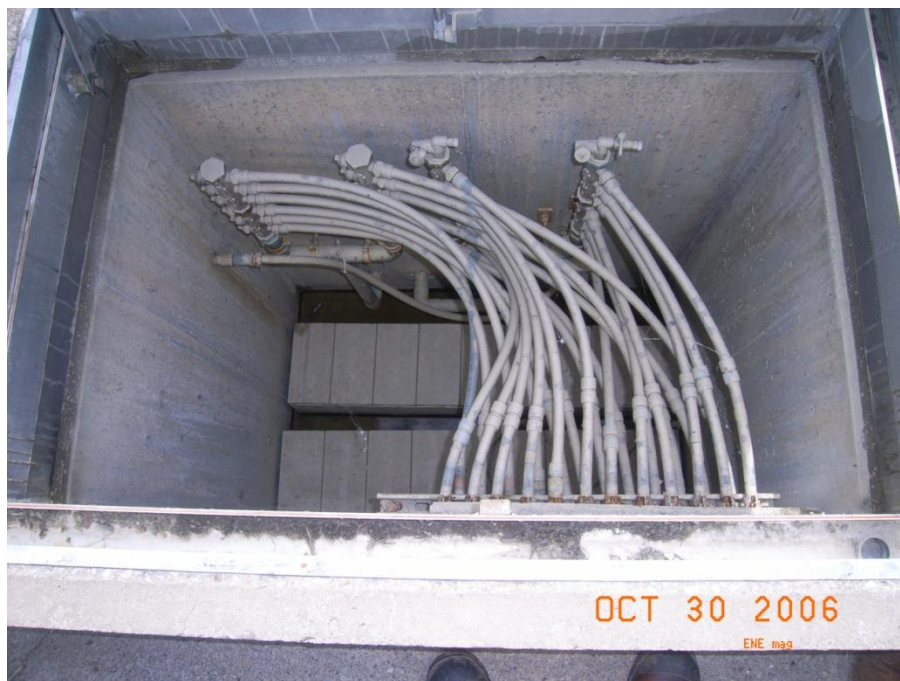
Controls for Heated Sidewalk (South end of Bldg at exit 15)
