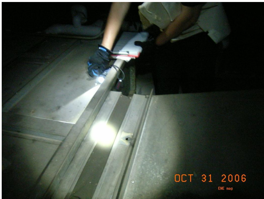
Vibration Dampening Material on Duct in Catwalk
