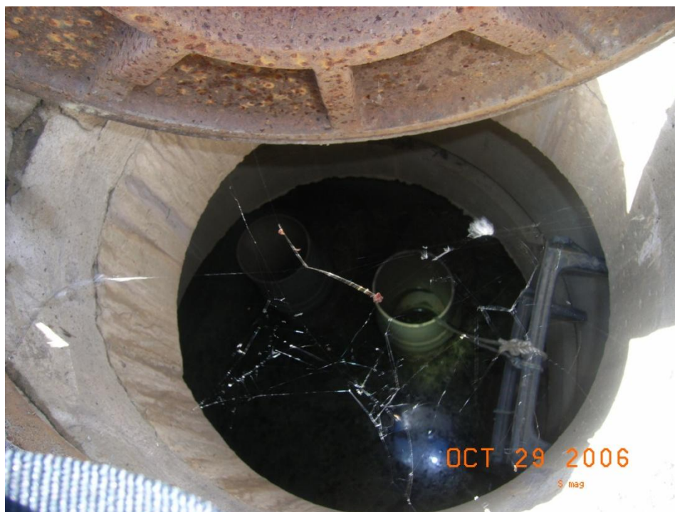
Oil Water Separator near Exit 16
