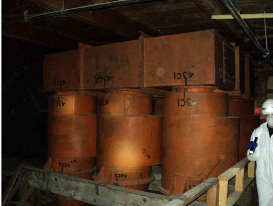
Metal Reclamation Units in Catwalk
