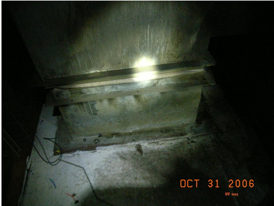
Vibration Dampening Material on Duct in Catwalk
