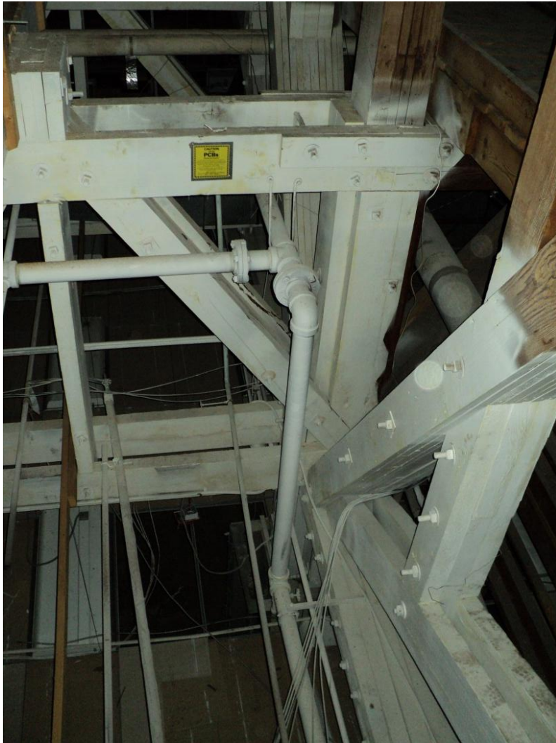
PCB Contaminated Beams and Columns in Catwalk (Painted)
