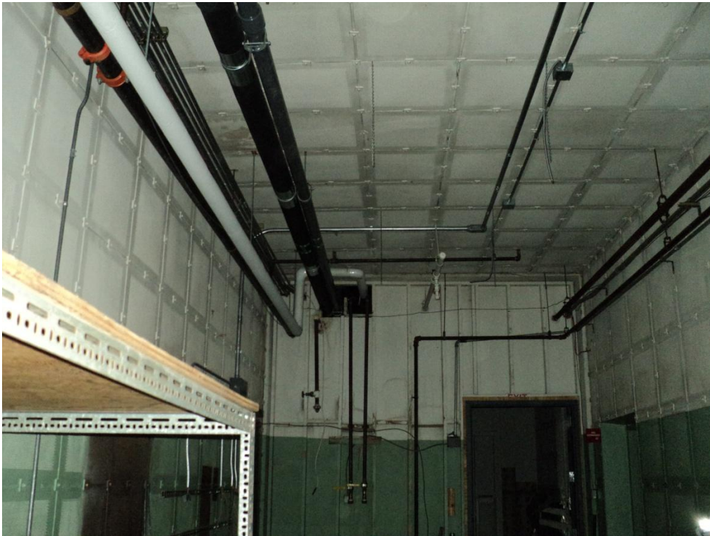
Range Building Control Room
