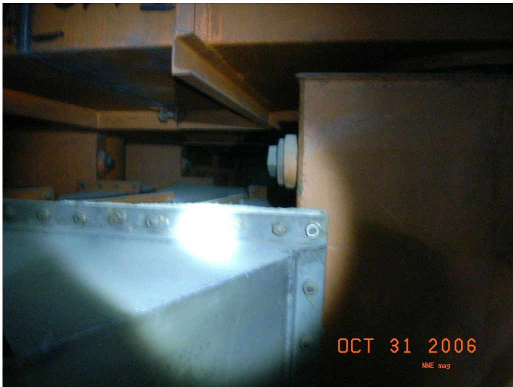
Metal Reclamation Unit on Catwalk (Suspect CWM gasket)
