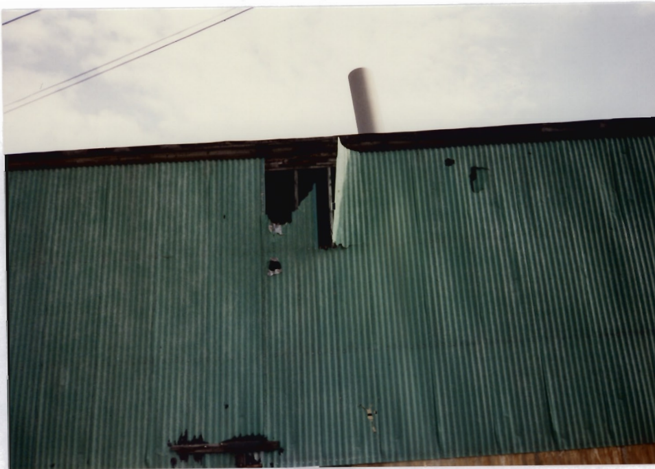
24. Continuation of photograph 23 showing the remains of the Fume Scrubber (SWMU 5). The view is facing east.
