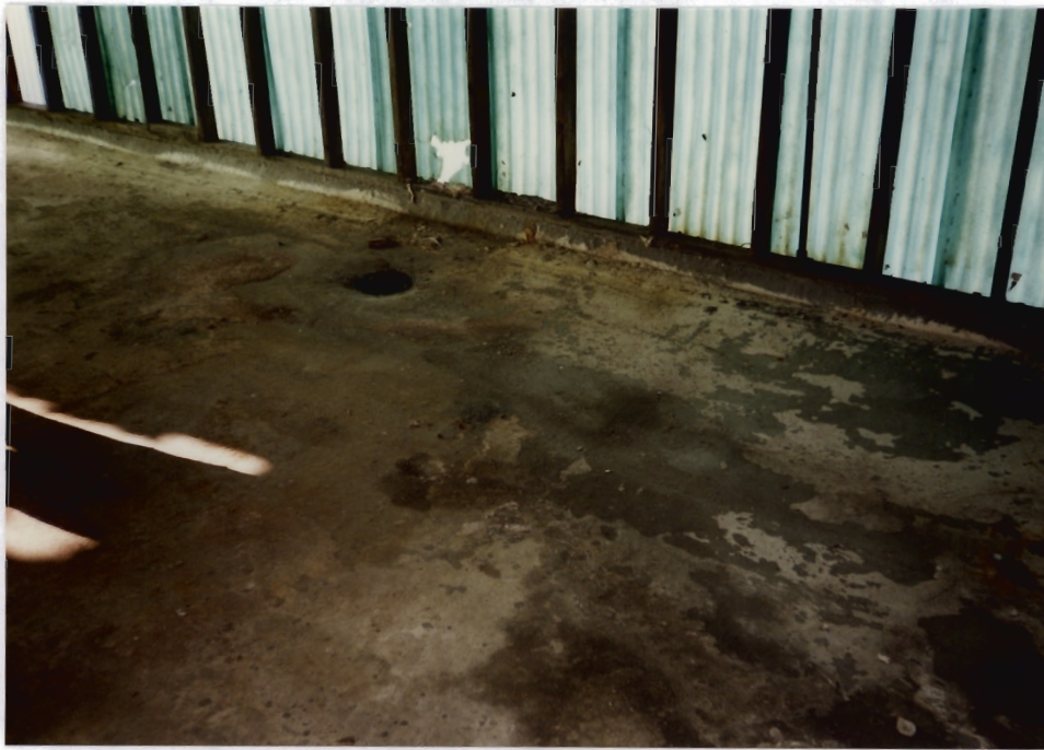
15. View of the immediate vicinity of the Barrel Wash Station (SWMU 4) showing a drain connected to the Process Sewer (SWMU 6). The view also shows the former location of the Fume Scrubber (SWMU 5).
