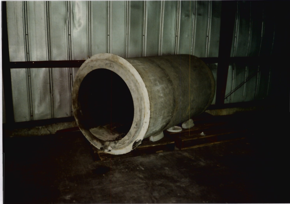
11. Interior view of Warehouse No. 2 showing the Solvent Recovery Sump identified as a SWMU in the PR. The sump was never used.
