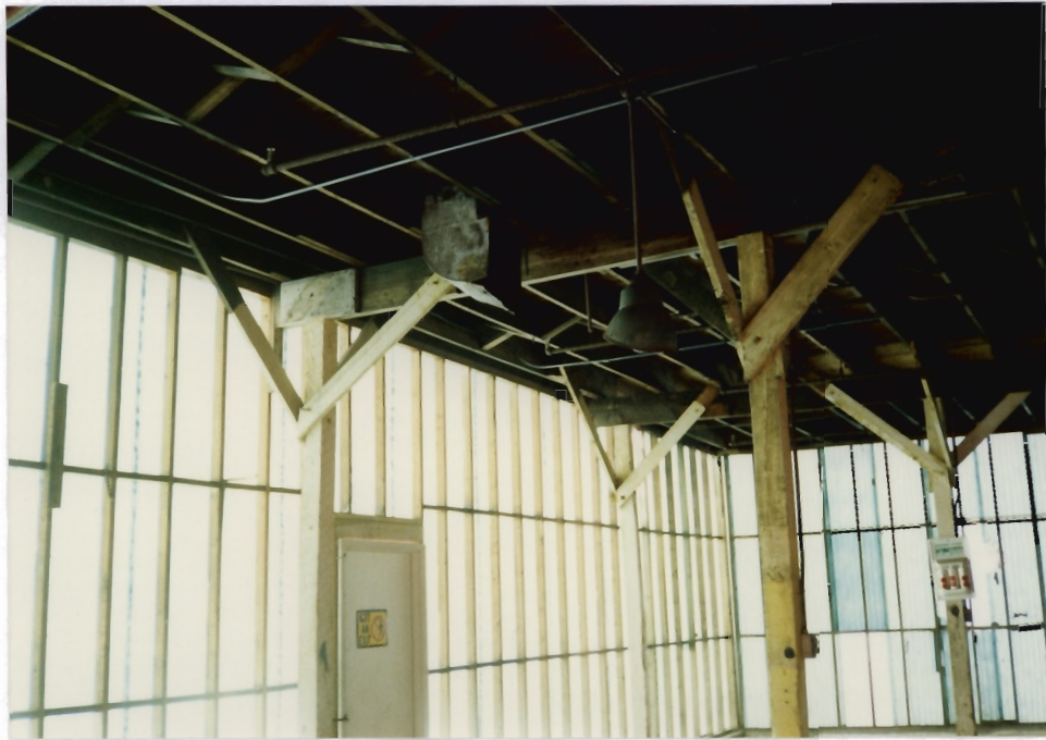
17. View inside Warehouse No, 3 showing a vent in the top of the photograph.
