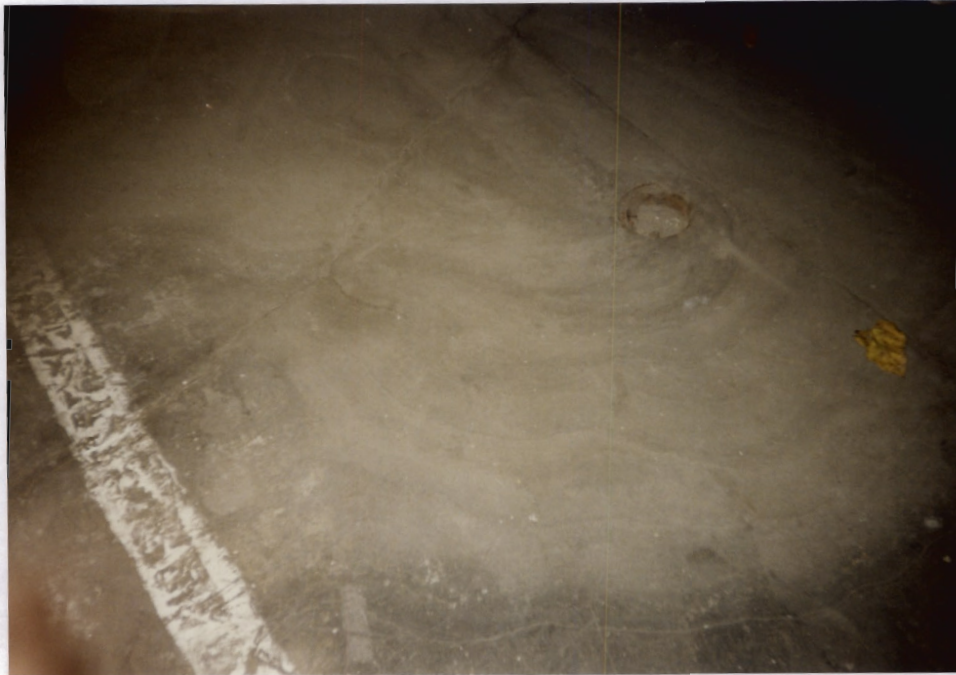
9. Close-up of the floor inside Warehouse No. 2 showing a Drain (SWMU 13). The drains inside Warehouse No. 2 were reportedly installed for drainage in the event the emergency fire sprinklers were used.
