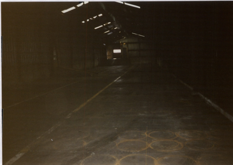
8. View inside Warehouse No. 2 located in the north section of the facility. The view shows the lower, product storage section of the warehouse. Note the rust stains in the foreground.
