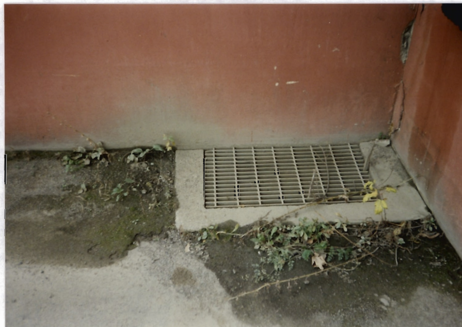
30. Close-up of a catch basin located outside Warehouse No. 4 in the southwest section of the facility.
