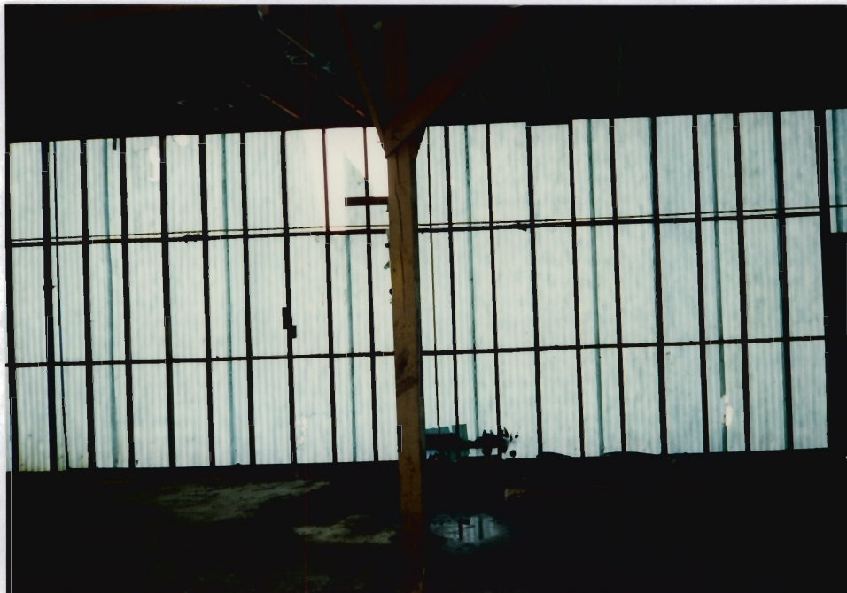
14. View of the Barrel Wash Station (SWMU 4) facing west. The current Neutralization Pit (SWMU 2) is located outside the green corrugated fiberglass wall shown in the center of the photograph.
