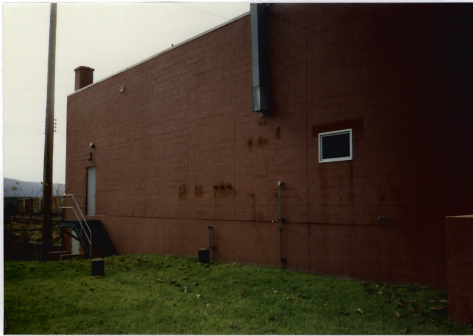
31. View of the east wall of Warehouse No. 4 showing the former intake lines from the Solvent Blend Tanks (Tks 101-103) in the center of the photograph. The view is facing southwest.
