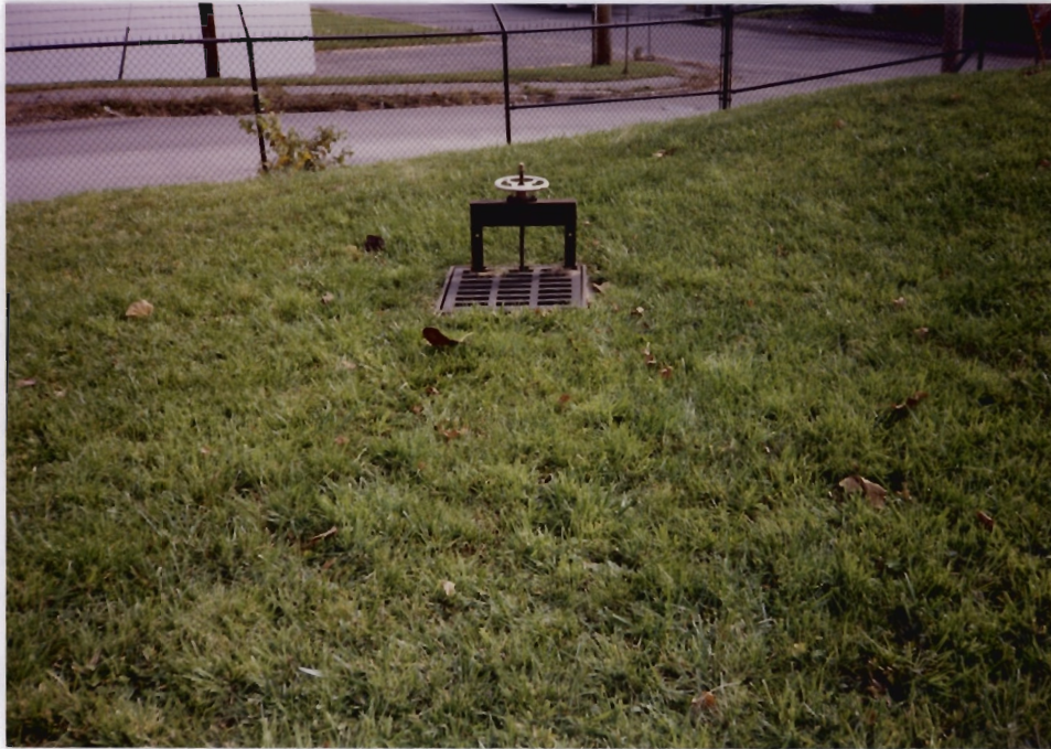
35. View of the emergency storm sewer control valve located in the southeast section of the facility.
