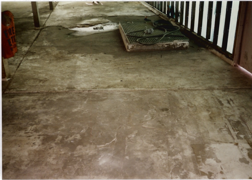
13. View of the Barrel Wash Station (SWMU 4). Note the eroded concrete filled with water in the top center of the photograph.
