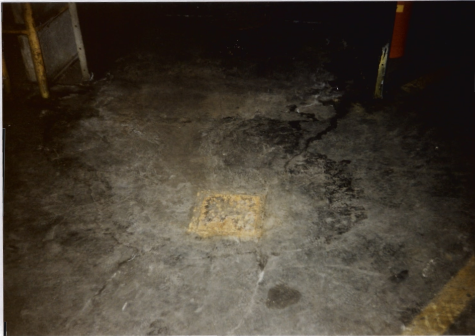
27. Close-up of a Drain (SWMU 13) in the vicinity of the paint booth shown in photograph 25. Note the stained floor.
