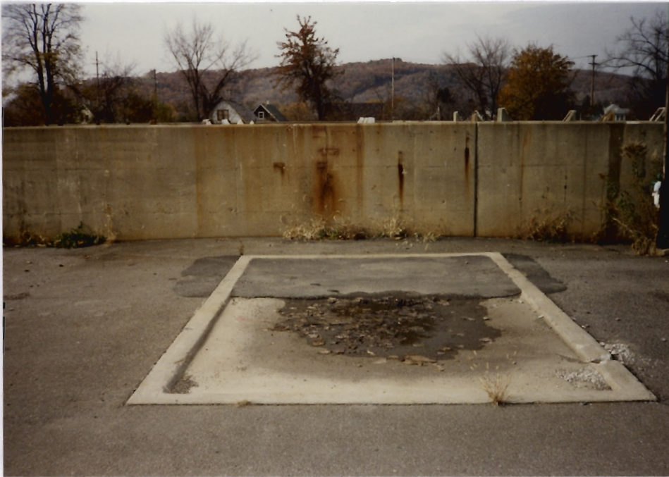
19. View of the Acid Truck Unloading Pad (SWMU 10) located in the vicinity of the Solvent Tank Truck Loading/unloading Area (SWMU 9) in the west section of the facility. The view is facing west. The former Acid Tanks (Tks 4-6), identified as SWMUs in the PR, were supported by the concrete structure shown in the background of the photograph.
