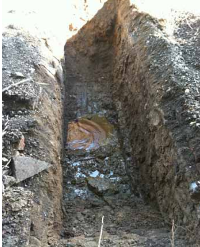
Photo #1 (2011.09.19): CTP1. Sheen/NAPL observed flowing in groundwater into bottom of test pit (looking south to north).
