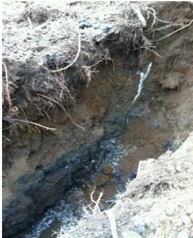
Photo #6 (2011.09.15): CTP-5. Gas holder #1 wall along east side of test pit at southwest end, NAPL blebs along bottom of test pit wall.
