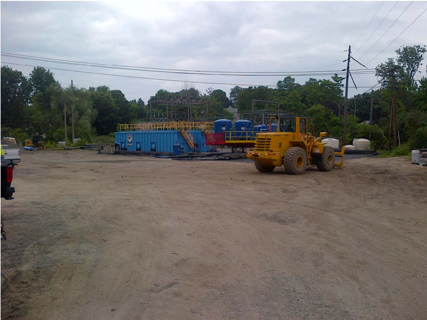
Wastewater treatment system and secondary containment
