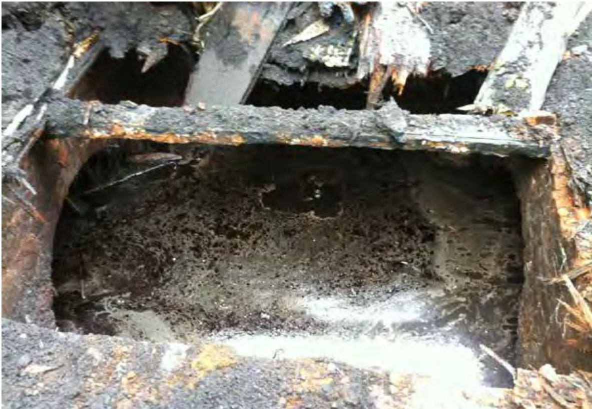
Photo #14 (2010.09.08): MTP-3B. Basement 'tunnel' filled with water, heavy NAPL precense.
