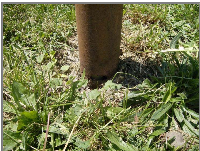
TW-5s has a rust hole at the base of the protective casing, not very visible in this photo, but the hole is oval-shaped, about two inches across.
