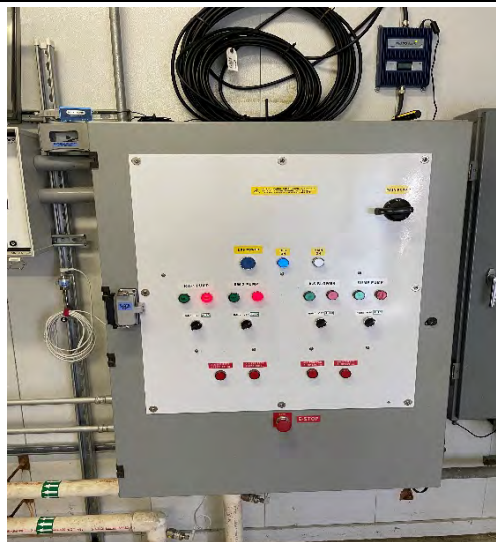
Exterior view of Main Control Panel (MCP).
