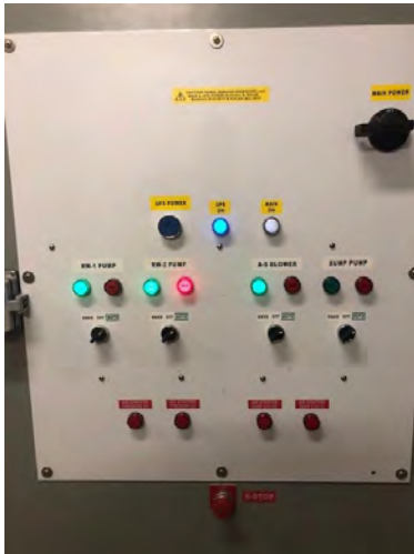
View of Main Control Panel door.
