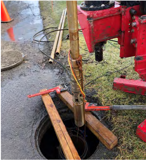
View of recovery well RW-1 pump removed from manhole.
