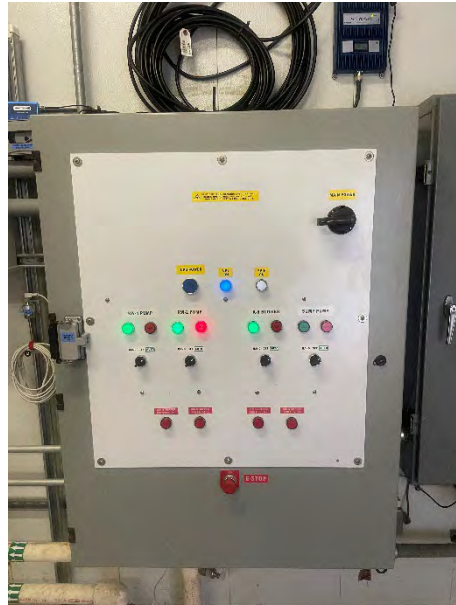
View of Main Control Panel door.
