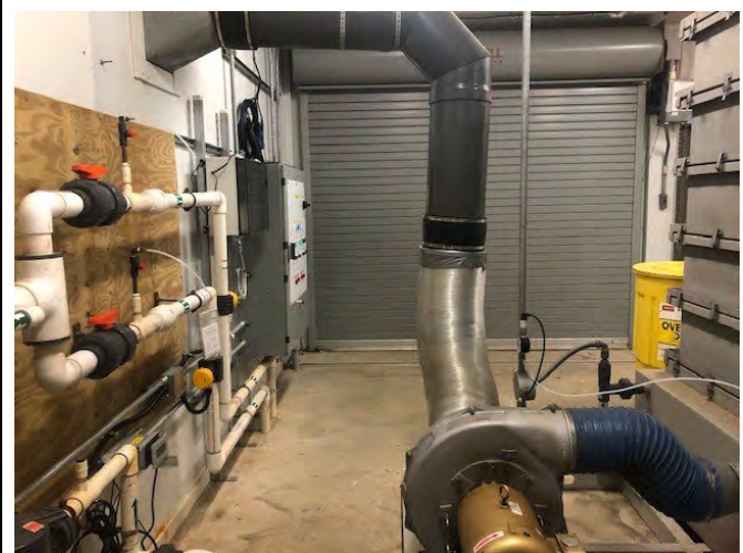
Interior view of treatment system building.
