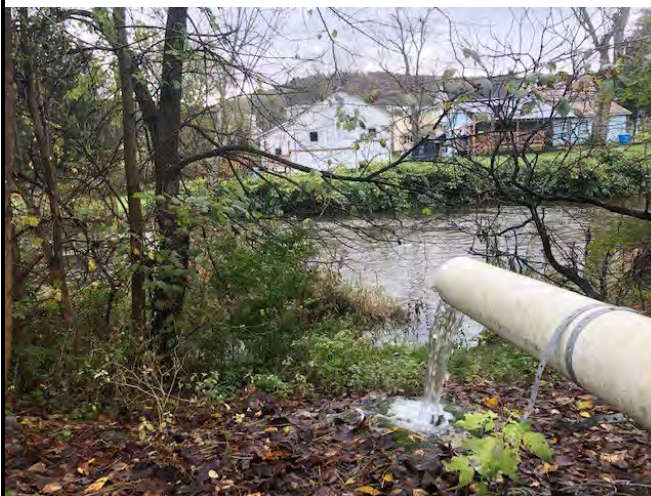
View of Effluent discharge to Otselic River.
