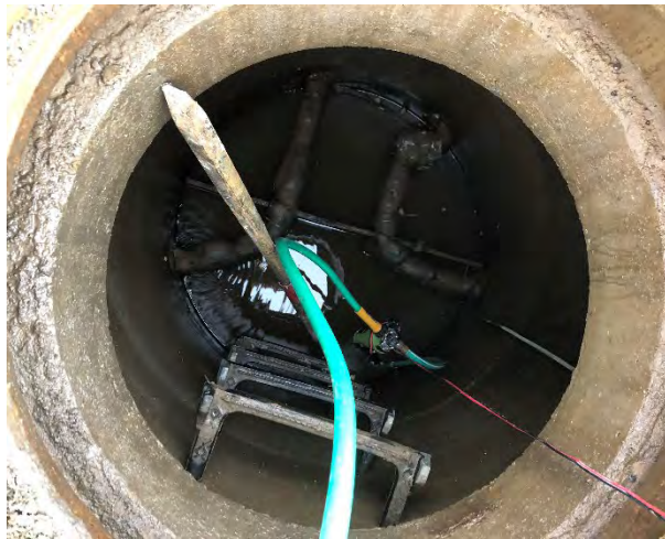
Pumping operations within recovery well piping manhole.
