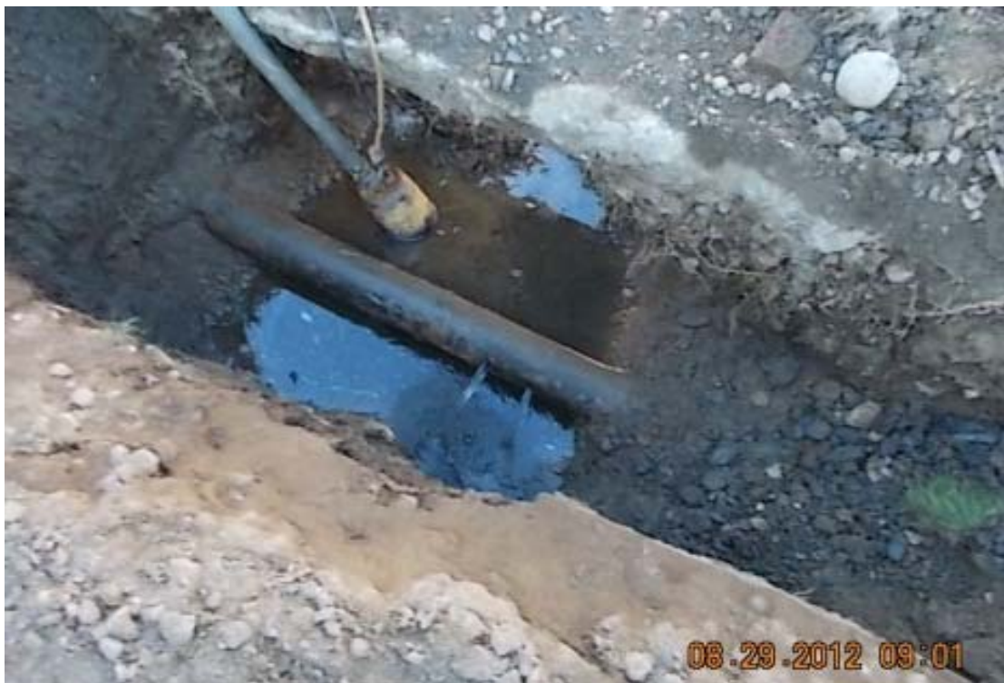
Photo #5: Leak in the northern portion of the original water main.
