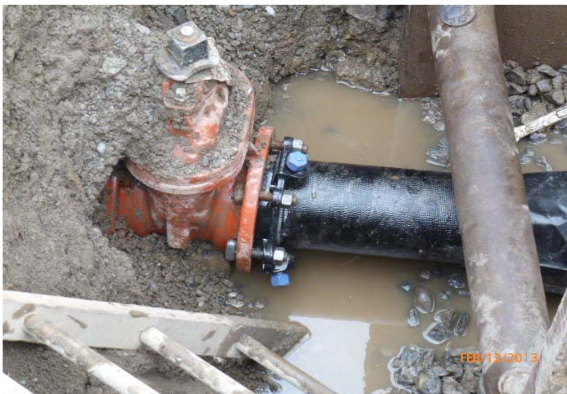
Photo #24: Water in trench at south end near Natoli's.
