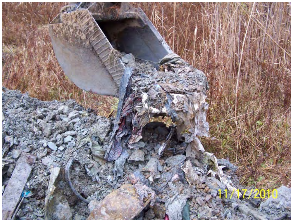
Photo 7579. Solid waste uncovered at TP-2, within 1 ft of the surface.
