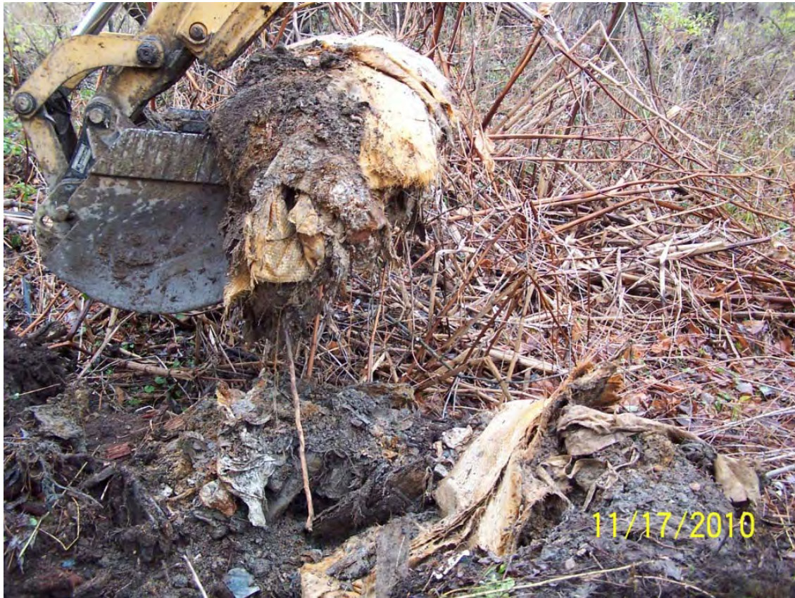
Photo 7595. Solid waste uncovered at TP-1D, which extended into the adjacent berm.
