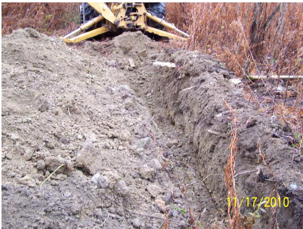
Photo 7613. No solid waste layer in TP-6, from toe of slope.
