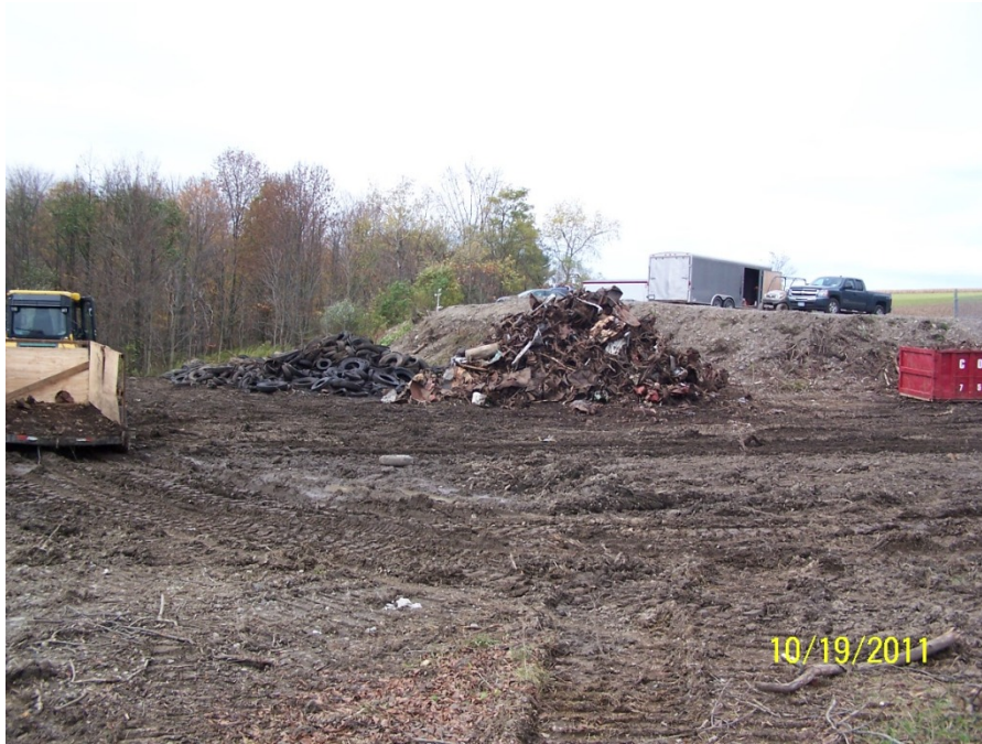
Scrap Metal and Tires Stockpiled Below the Toe of Slope of the Parking Area, Looking Northwest
