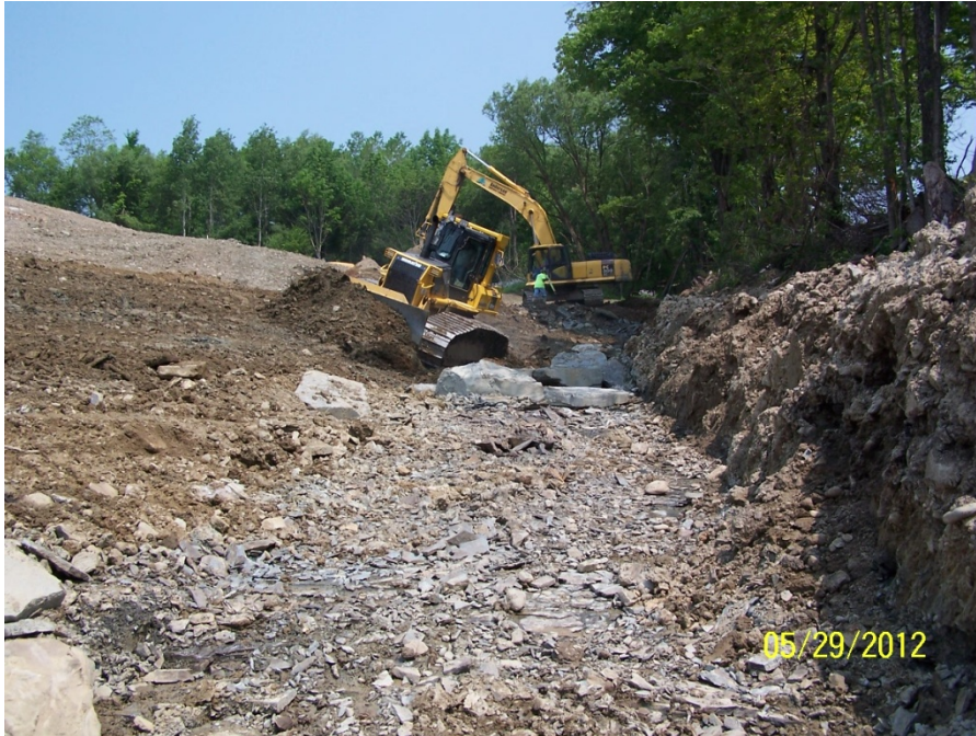
Southern End of the Eastern Perimeter Road Excavated to Weathered Shale, Looking North
