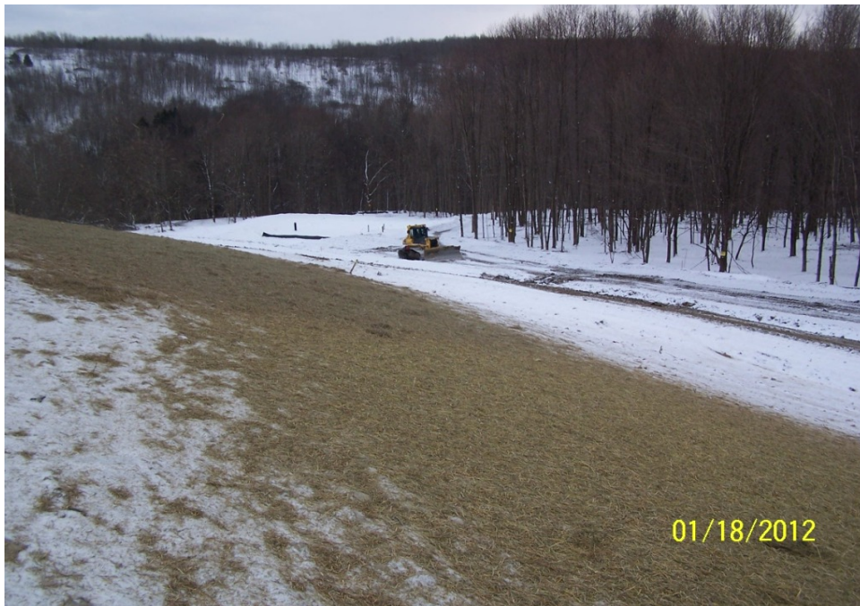
Solid Waste Covered with Six Inches of Select Borrow and Hay for Winter Shutdown, Looking Southeast
