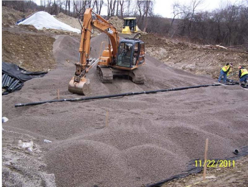
Installing Crushed Stone and Underdrain Piping at the Sedimentation Basin, Looking Northeast
