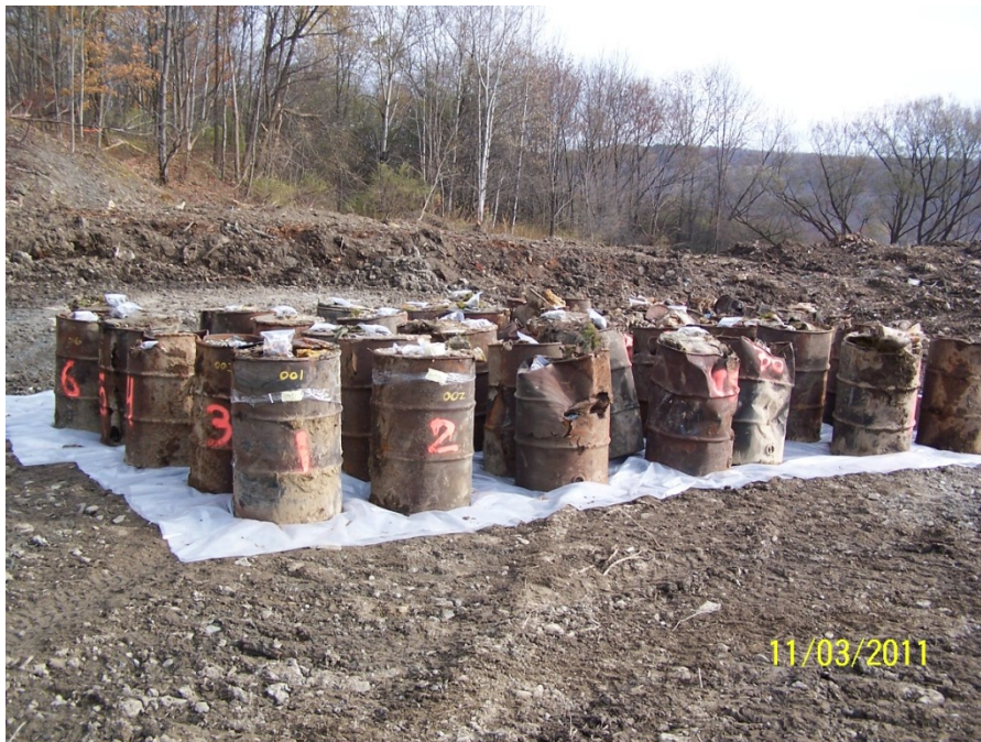
Drums Staged on Plastic for Off Site Transportation and Disposal, Looking Northeast
