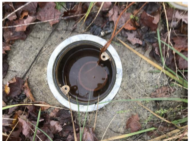
Flush mounted monitoring well
