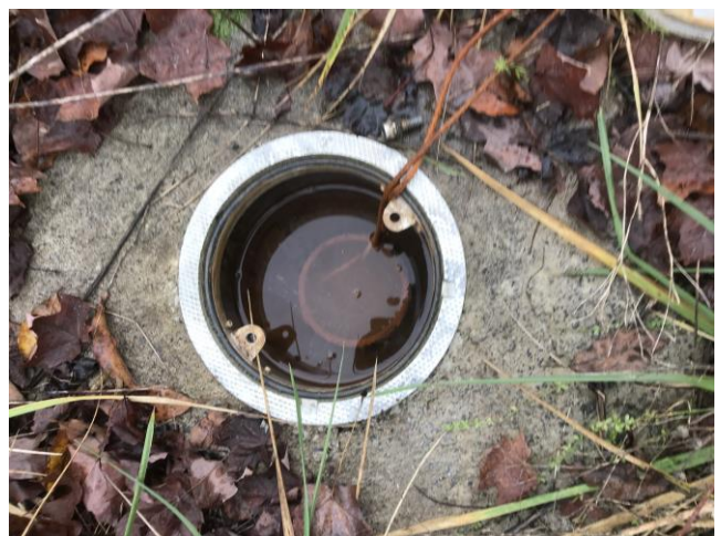
Flush mounted monitoring well
