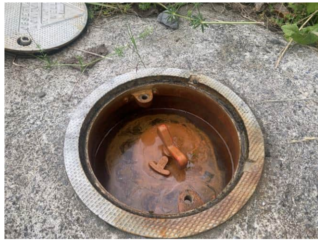
MW-3BR2 experiencing upwelling of groundwater. High iron content makes it appear like leachate, but no odor.
