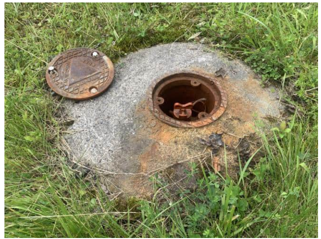
MW-3SR2 experiencing upwelling of groundwater. High iron content makes it appear like leachate, but no odor.
