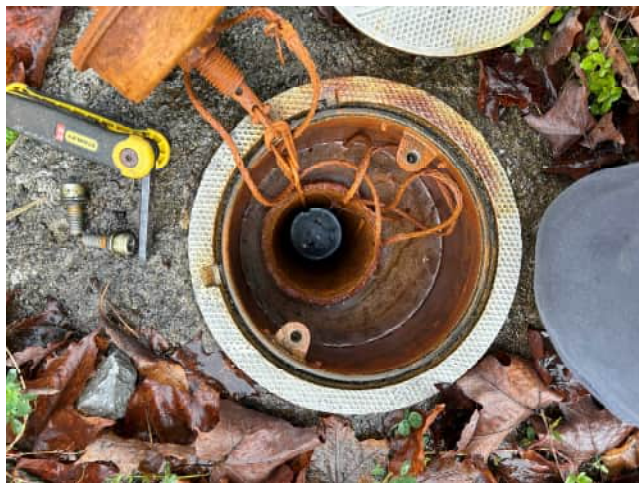
MW-3BR2 covered in leachate seepage.
