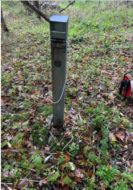
MW-1S has a cracked curb box.
