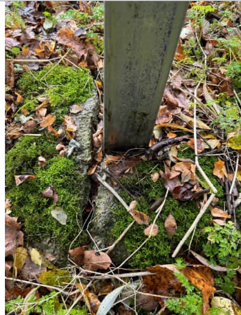
Close up of the cracked curb box.
