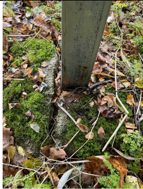
Close up of the cracked curb box.
