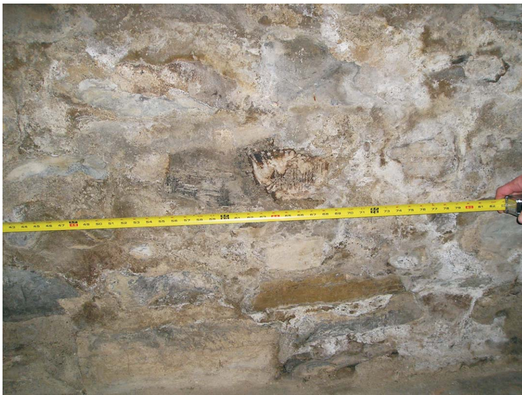
Photo #20: Stone #1 after sampling. Located approximately 5 feet from the wooden partition wall.
