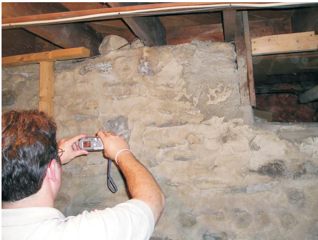
Photo #19: Background (Scrape #3) locations on south basement wall. Note crawl space access in upper right corner of photograph.
