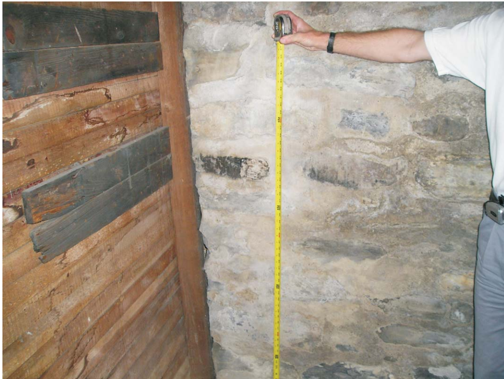
Photo #22: Stone #2 after sampling located approximately 3.5 feet above basement floor. Stone #3 is to the right of the measuring tape.
