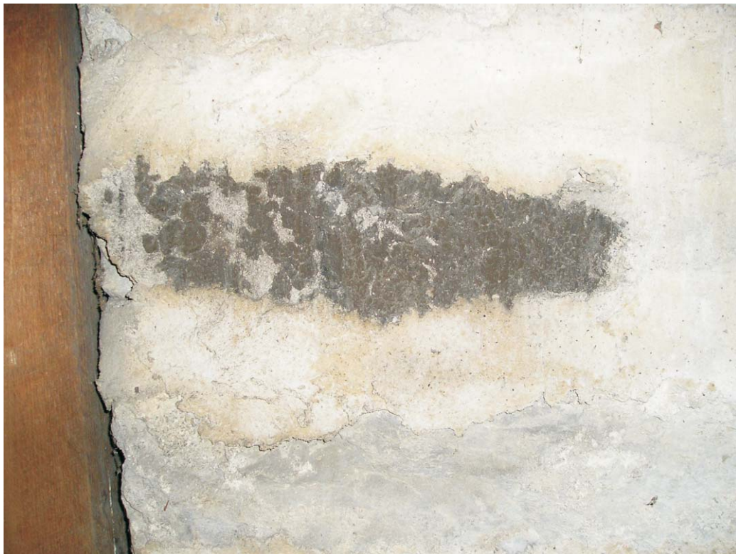
Photo #14: Stone #2 prior to sampling. Note crackly appearance.
