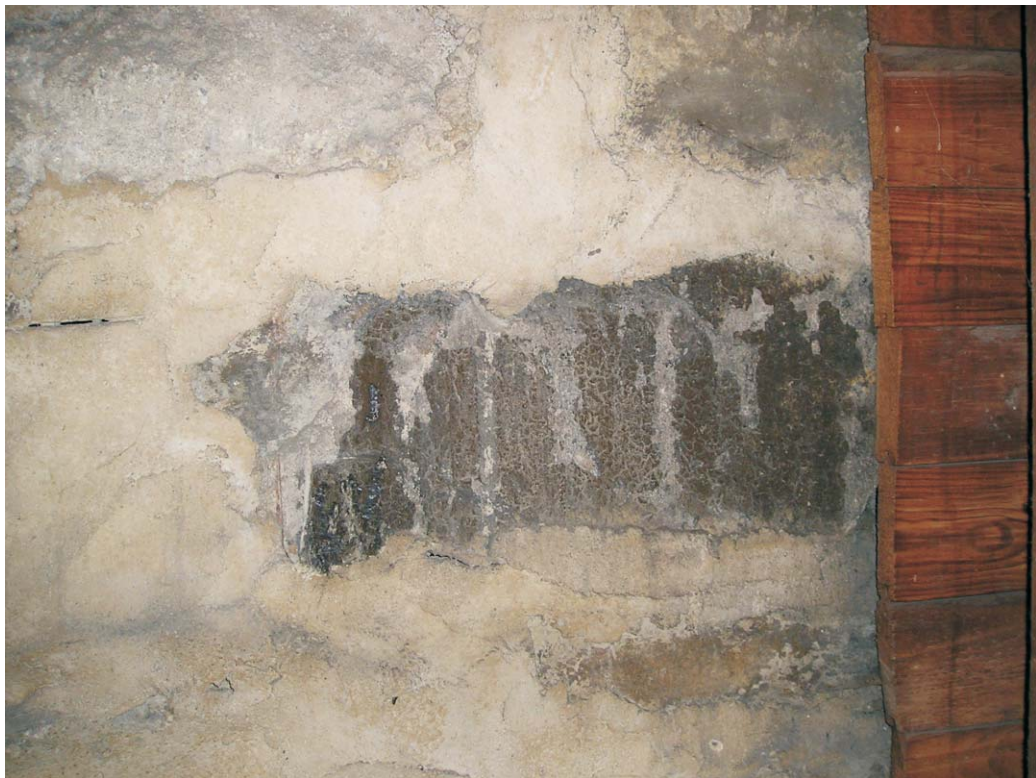
Photo #16: Stone #4 with black crackly appearance prior to sampling.
