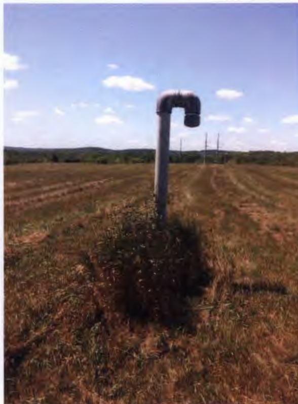
Photo 4. Gas vent V-11 with tall grass growth – August 2016.
