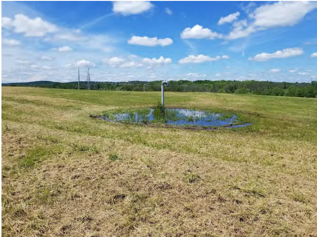
Photo 8. Ponded water in settled area at vent V-5. To be repaired during solar panel construction. . – June 2019.
