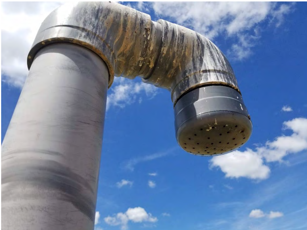
Photo 4. Gas vent screen is clear of blockages allowing gas to vent properly – June 2019.
