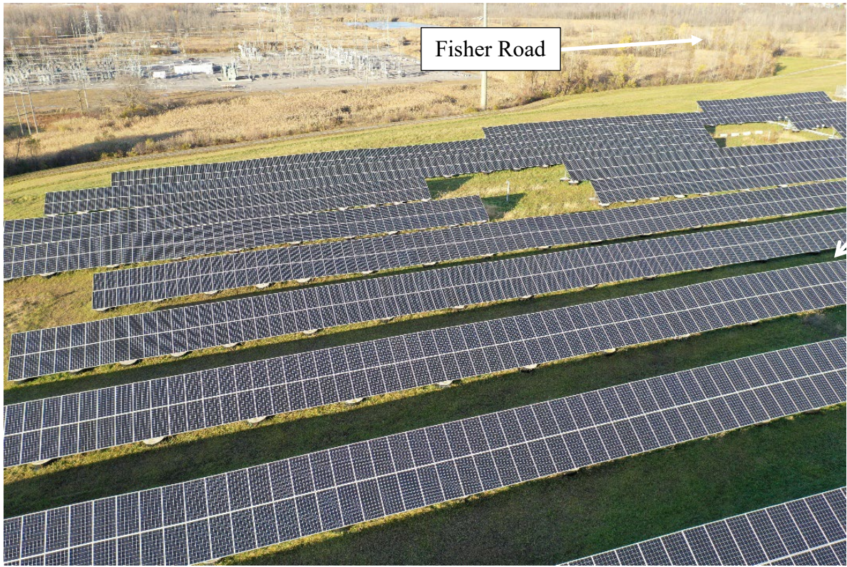
Photo 7. Viewing NE at solar panel array. November 2021.
