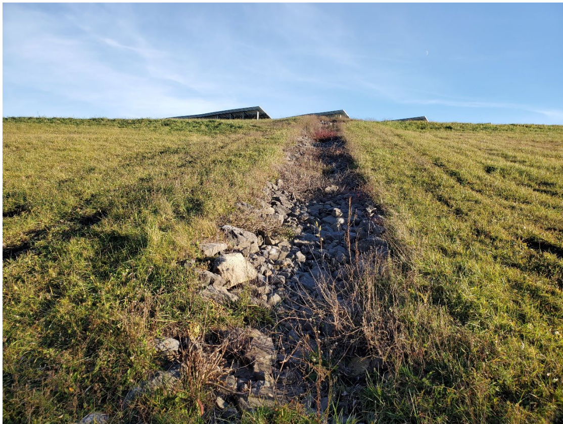
Photo 6. Down chute on NW corner of landfill is open and clear. Solar panels in background. – November 2021.
