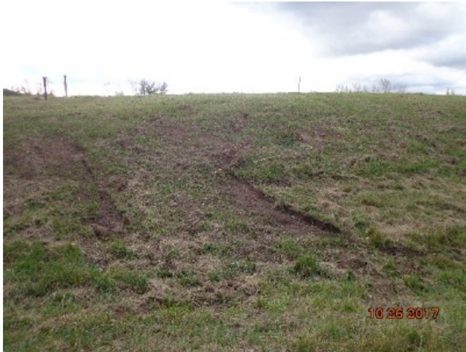
Photograph Number 7: Representative view of isolated rutting following annual mowing.
