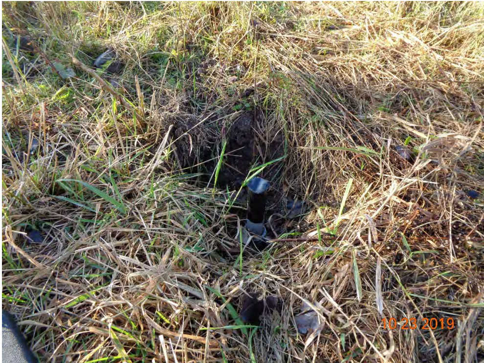
Photograph Number 15: View of damaged W-10.2 with no protective casing or concrete pad and apparent broken PVC riser. Unknown cause of damage.
