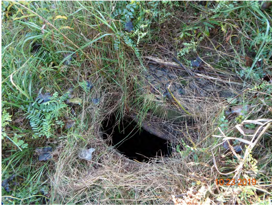
Photograph Number 7: View of manhole with cover and frame displaced.
