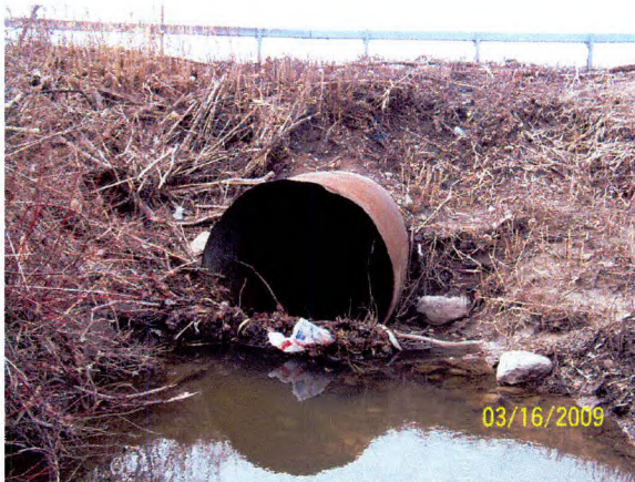
88 Culvert at Mautz Road looking west — no concrete collar around culvert
