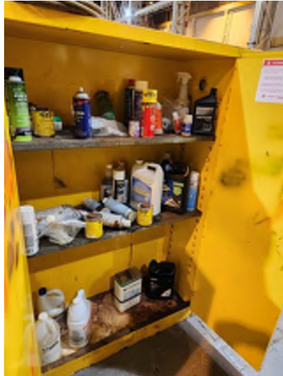
Photo Title: 20221221_160945.jpg Date: 12/21/2022 Description: Flammable storage cabinet in TR-5 warehouse area.
