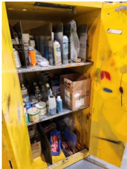
Photo Title: 20221221_161007.jpg Date: 12/21/2022 Description: Flammable storage cabinet in TR-5 warehouse area.
