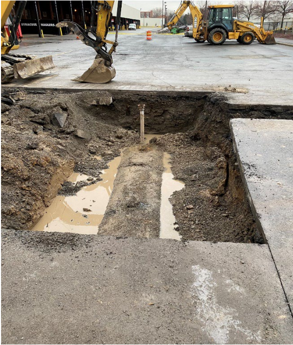
1 - TOP OF TANK EXPOSED IMG_6057
