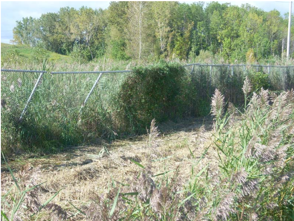
Photo 6: View of downed fence along Factory Avenue facing southwest.
