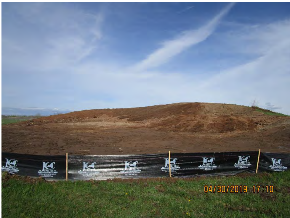
Berm completely collapsed and graded
