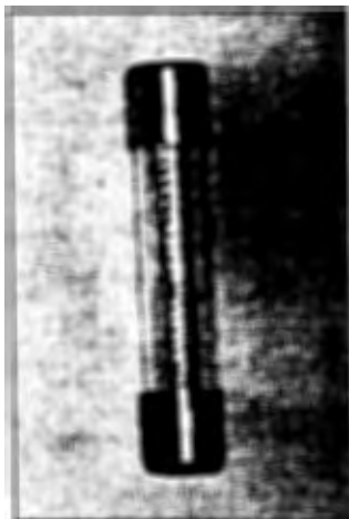
The fuse removed from the holder. Always replace with the proper part; 7.5 Amp Slow-Blow.
