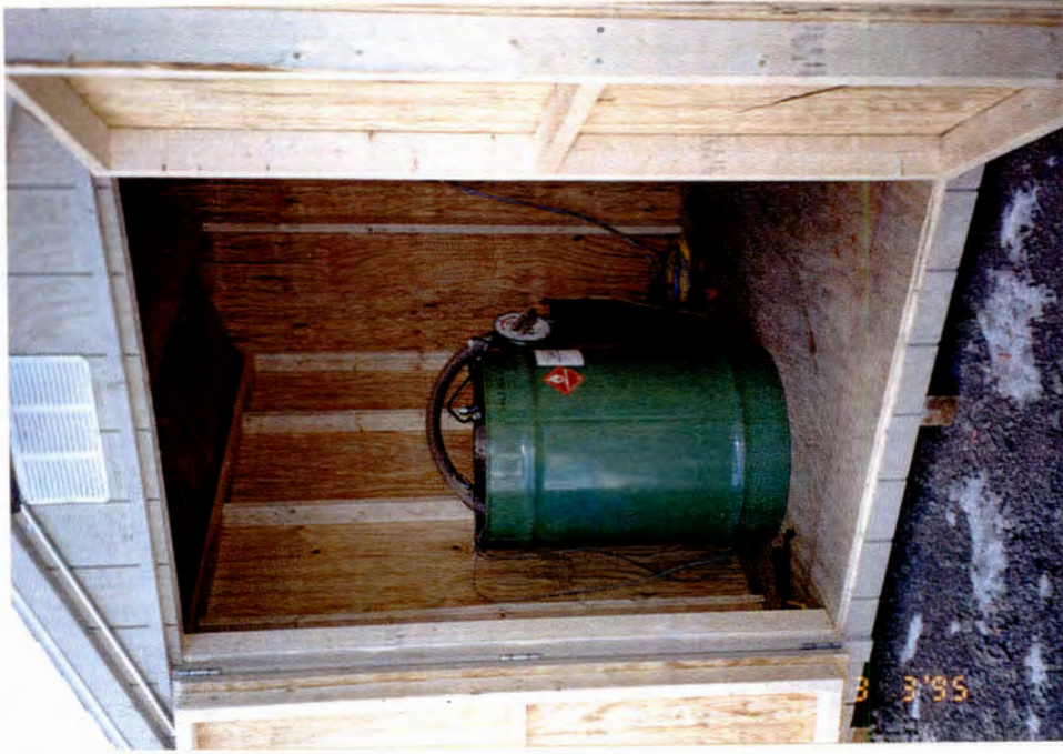
1) Building showing product storage drum and ALS on well head.
